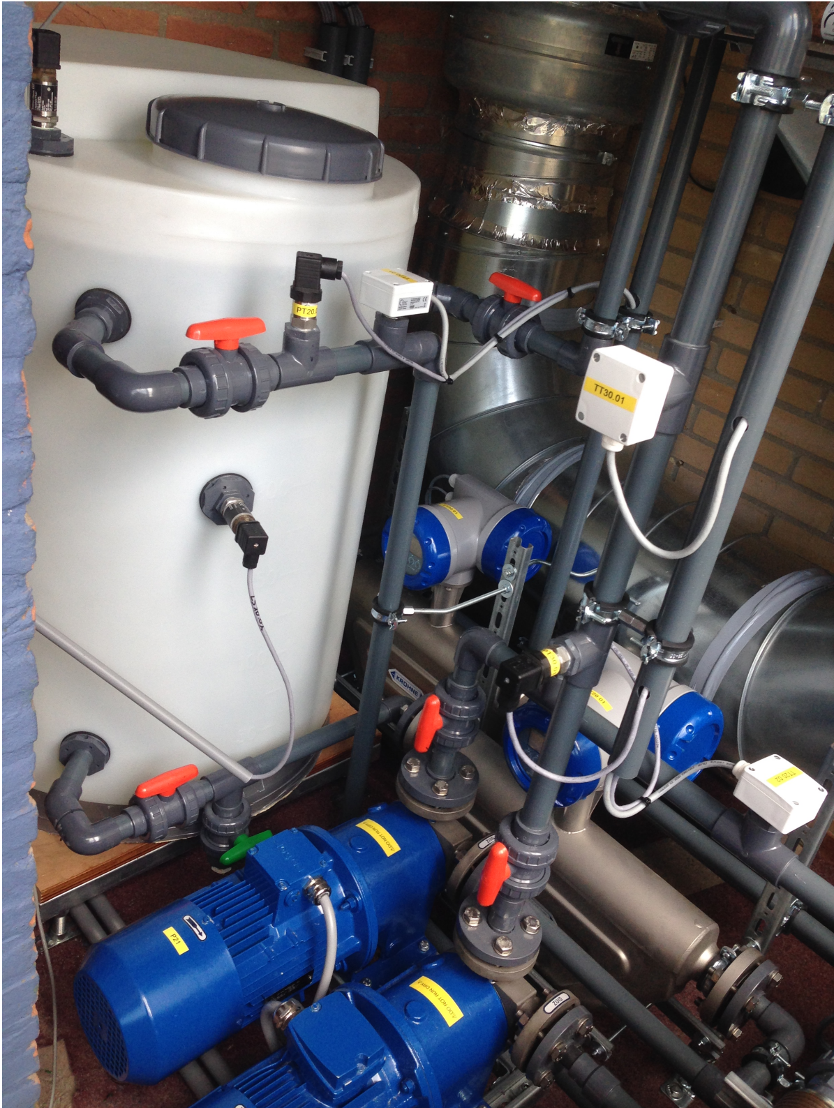
Figure 5.2: The pilot system in Twello before the insulation was installed. The white vessel is the storage tank which is connected with the grey tubes to the other components. The airducts is shown in the background; it has a number of bends which are include in the pressure drop calculations. The black sensors measure the gauge pressure; notice how some sensors are placed much further from the ground than others.
