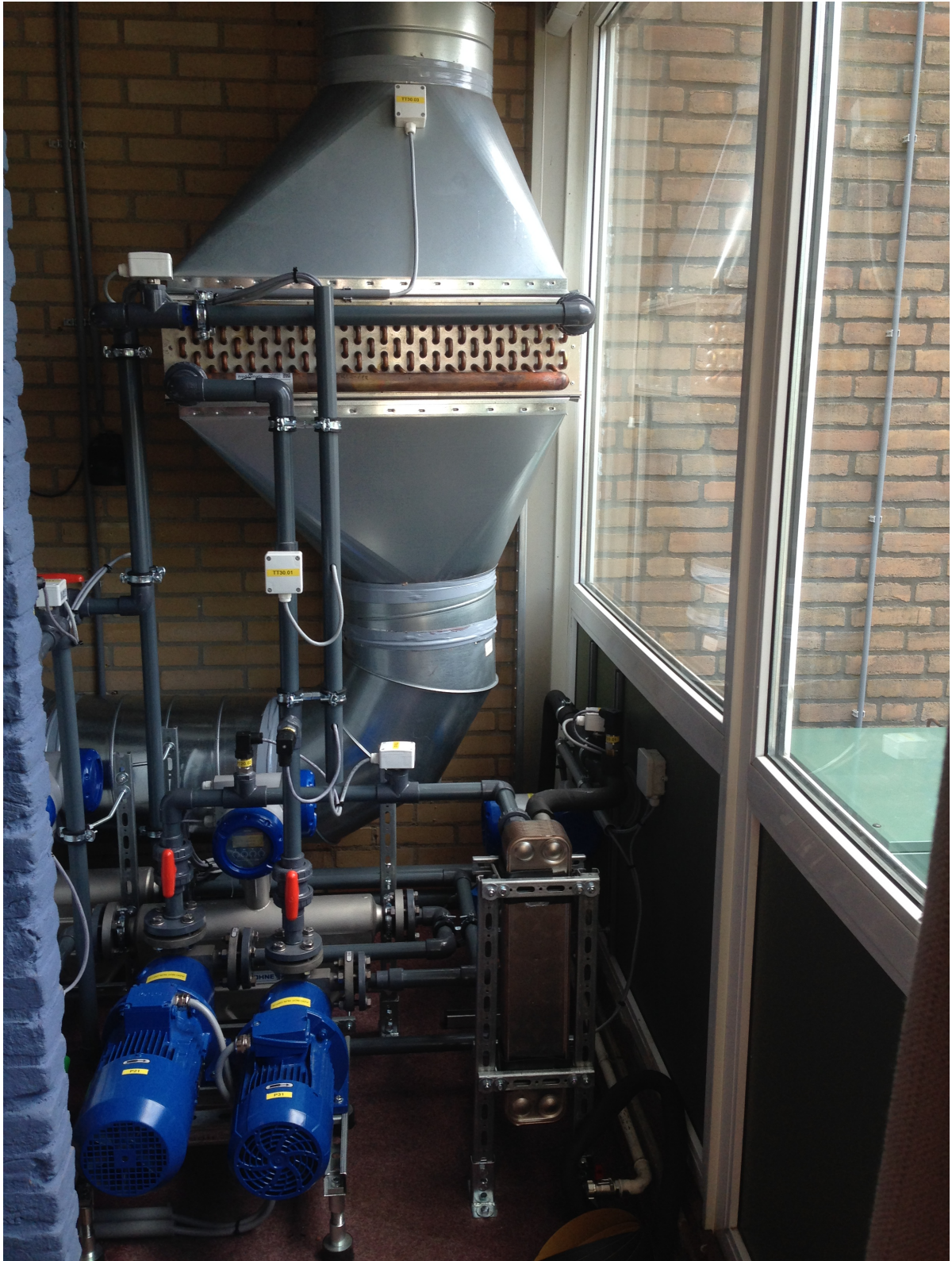
Figure 5.1: The pilot system in Twello before the insulation was installed. In the top the air cooler can be seen. It is connected the other components with the grey tubes. Pleas notice the sensors implemented in the system. These sensor are not necessarily placed at the in- or outlet of the components.
