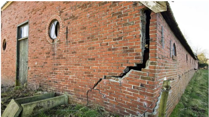
Figure 1.29: Subsidence due to dry summers (BNNVARA, 2019)
