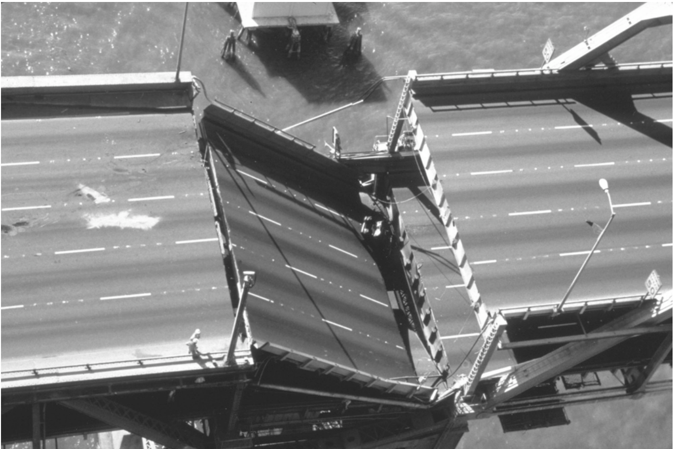
Figure 7.3a | Loma Prieta Earthquake damage on Bay Bridge, in Northern California on 17 October, 1989 [5]
