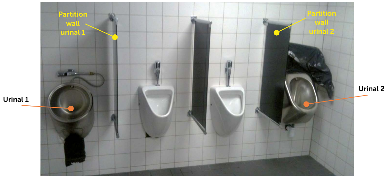
Figure 6.6 Test setup in male lavatory.
