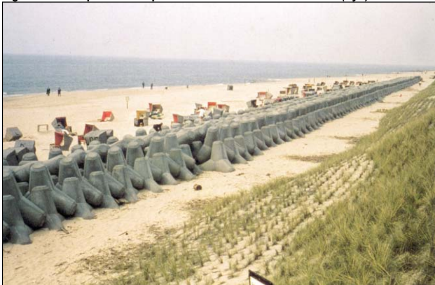
Figure 4-2 Example of a tetrapod dune foot revetment at Hörnum (Sylt)
