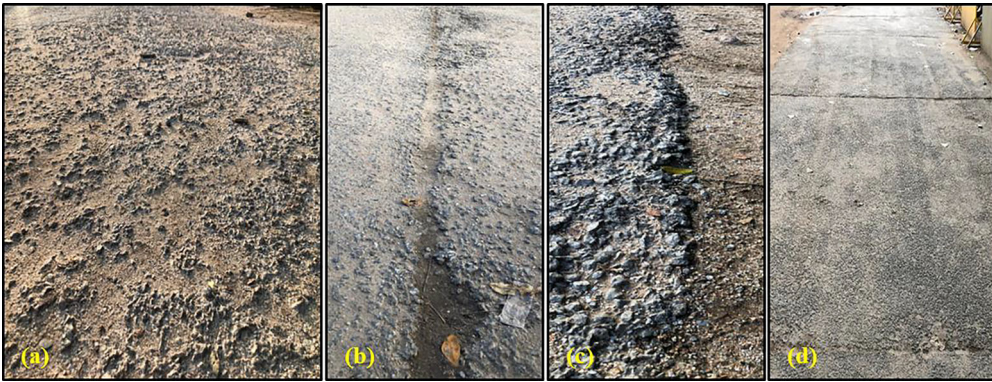
Figure 3. Structural defects: (a) severely ravelled pervious concrete pavement slab, (b) joint deterioration, (c) edge cracking and (d) skid marks.
