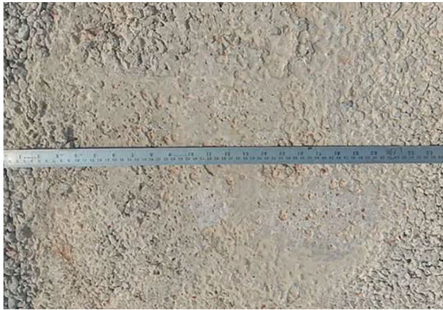
Figure 4. Severely sealed surface of pervious concrete pavement slab.
