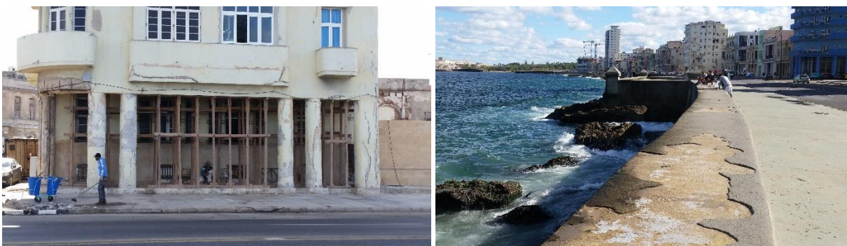
Figure 8: (a) Damaged building behind the Malecón (left), (b) example of an outcrop (right)
