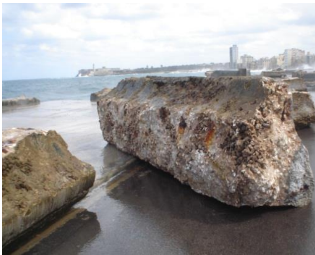
Figure 15: Structural failure of the sea wall during hurricane Wilma
