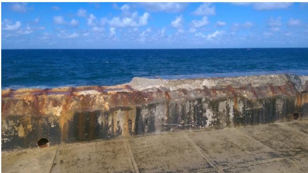
Figure 10: Large segment of crest missing with corroded reinforcement
