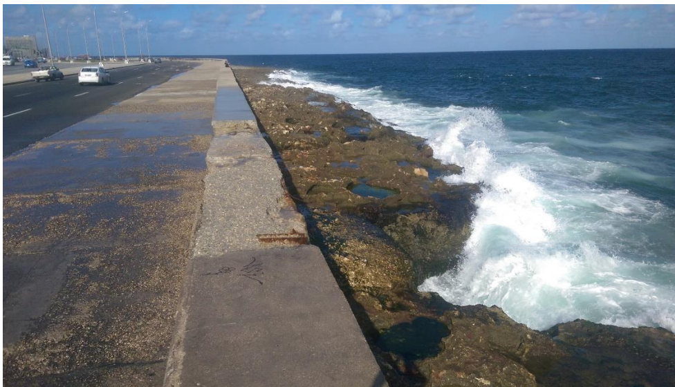
Figure 14: Drain entrance in the sea causing additional overtopping and structural damage
