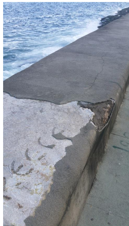
Figure 13: Damage to the outer layer in section 4 and 5
