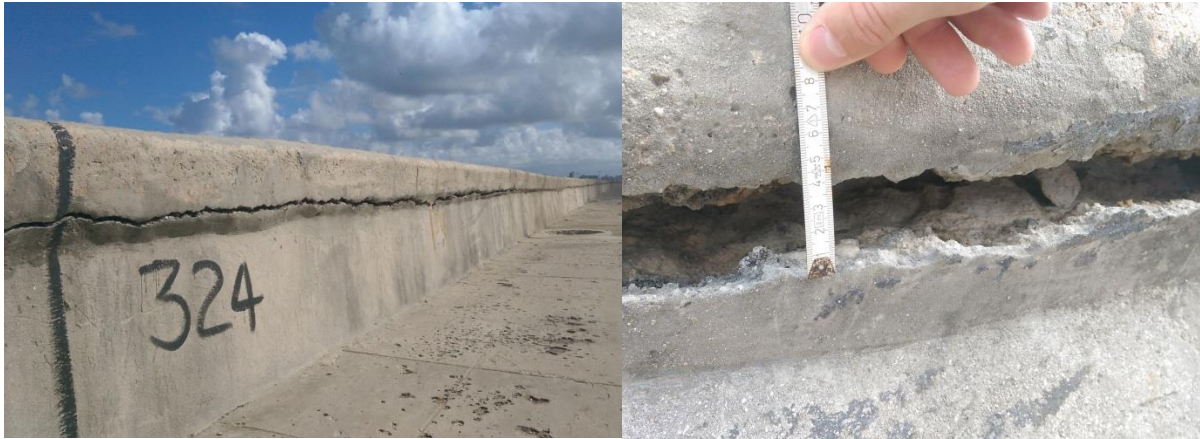
Figure 11: Longitudinal cracks in section 2 near Calle B and C
