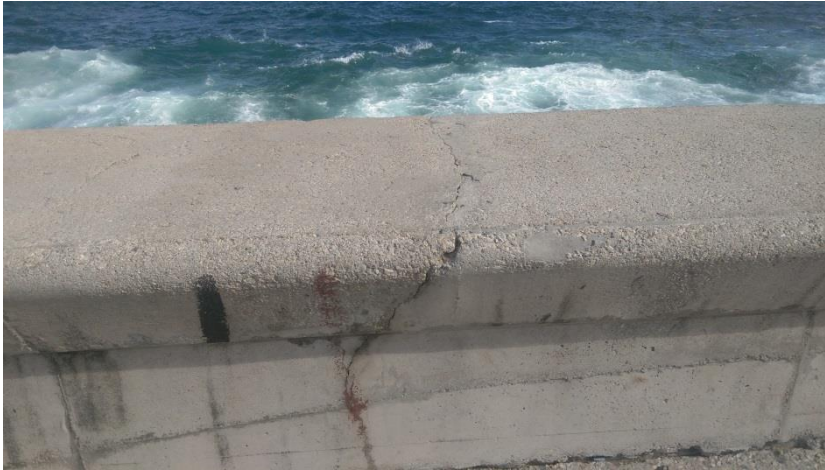
Figure 12: Large transverse crack crossing the crown into the seawall
