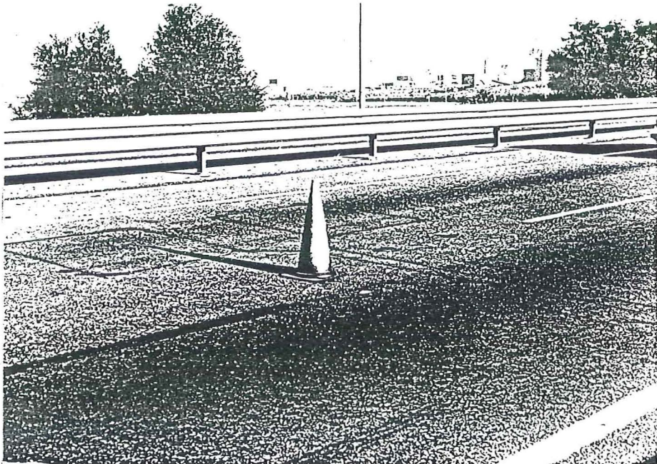
Photograph of installed inductive loops
