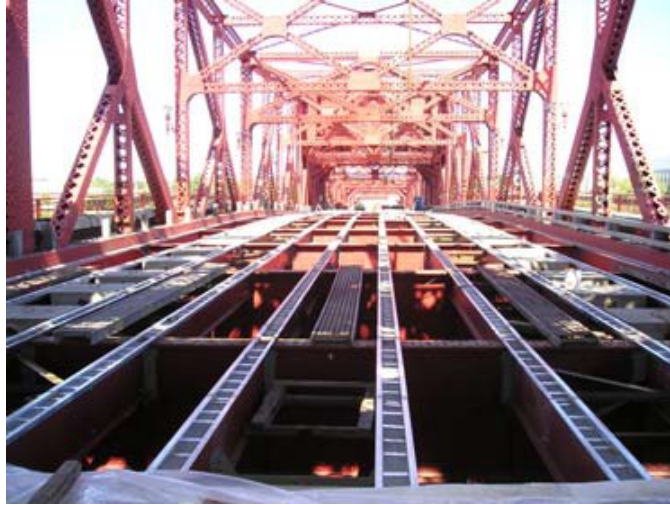
Figure 2-85 The Bridge's longitudinal stringers were prepared for placement of FRP panels (Sams, 2005)
