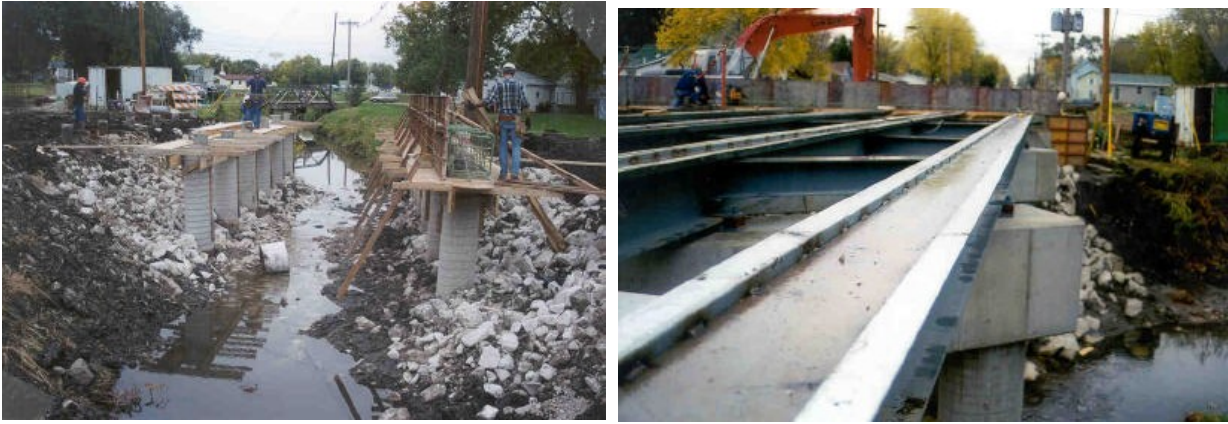
Figure 2-68 Concrete Encased Metal Shell Piles (left) and Angle Irons Tack Welded to the Girder Top Flange (right) (Winkelman, 2002)
