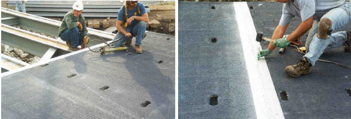
Figure 2-71 Compression of the Field Joints with Hydraulic Hand Jacks (left) and Composite Doweling of the Field Joints (right) (Winkelman, 2002)
