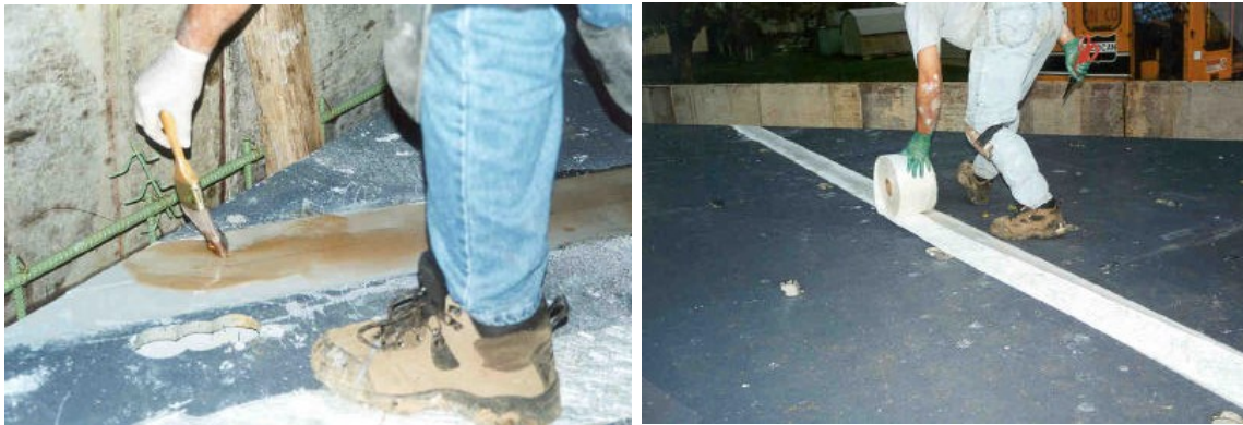
Figure 2-74 Vinyl Ester Resin Application to Field Joint (left) and Composite Material Strip Used over Field Joints (right) (Winkelman, 2002)
