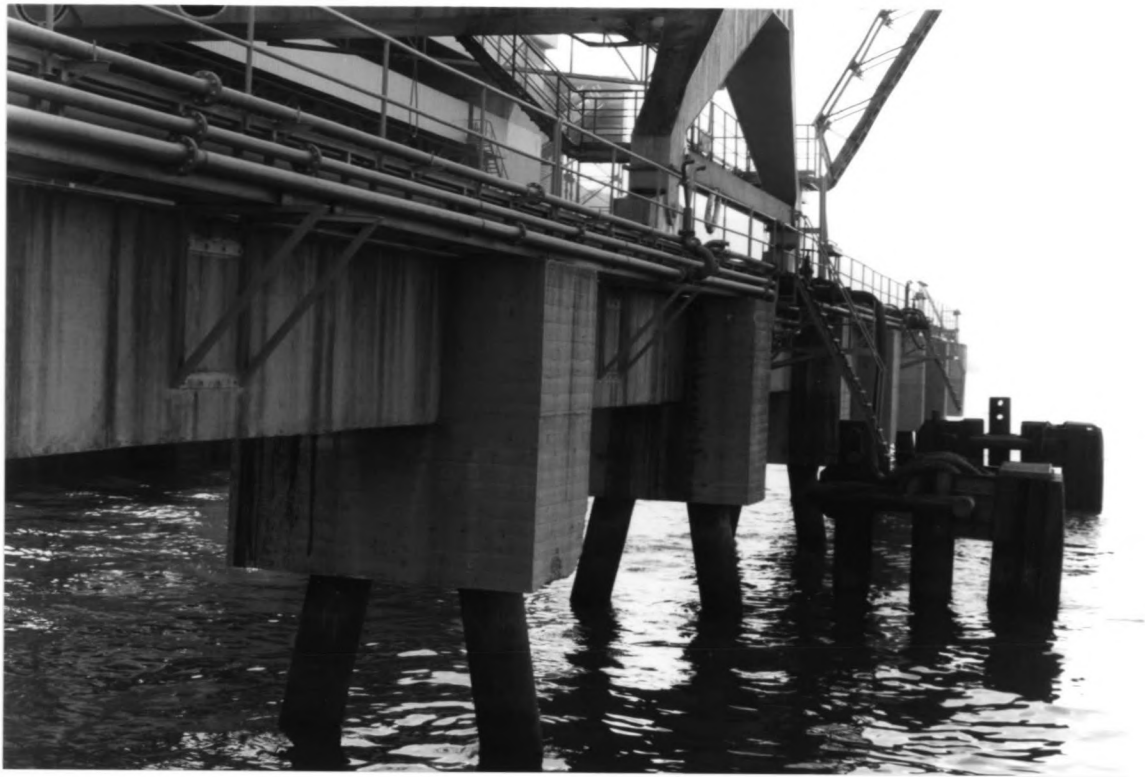
LOADING BERTH TAGOL (PICTURE 13)
