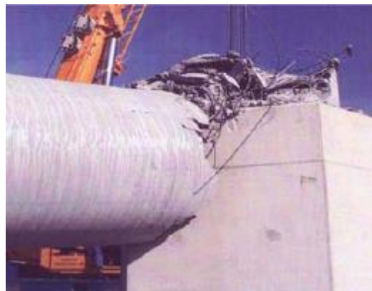
Figure 2.2: Concrete wind turbine after collapse due to concrete compressive fatigue (Van der Veen and Den Uijl, 2015).
