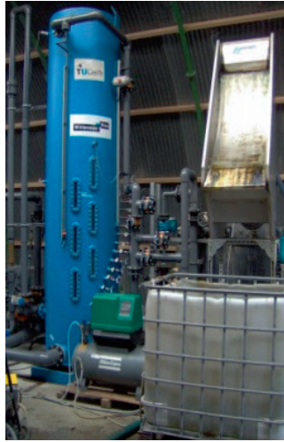
Figure 3.2 – Multi media filter at the WWTP Horstermeer
