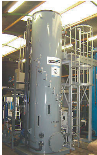
Figure 3.3 – One Step Effluent Polishing (1-STEP ® ) filter at the WWTP Horstermeer
