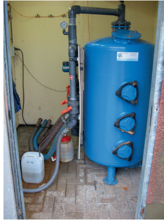
Figure 3.7 – Granulated activated carbon filter at the WWTP Maasbommel
