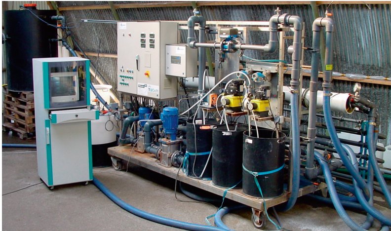
Figure 3.4 – Ultrafiltration pilot installation at the WWTP Horstermeer
