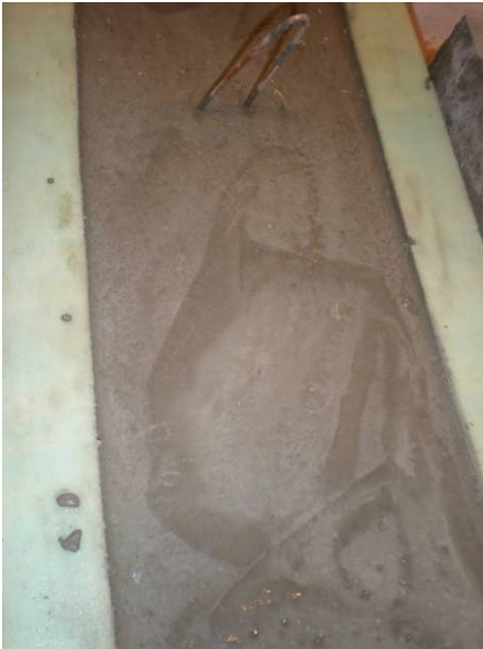
Figure 8-35: Deformed concrete, top side
