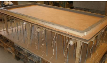
Figure 10-8: Strings at the edge to be able to take the tension forces at the edge supports
