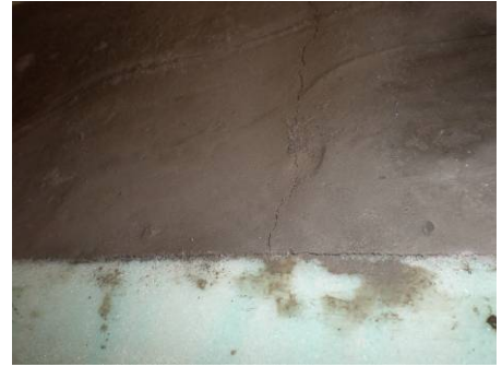
Figure 8-27: Crack, element in mould, top
