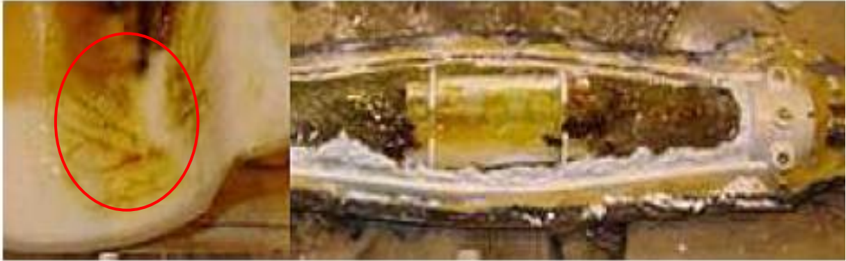
Figure 2.8: Fluid filled joint from a certain circuit containing electrical tracking marks (left) and probable moisture ingress [14].
