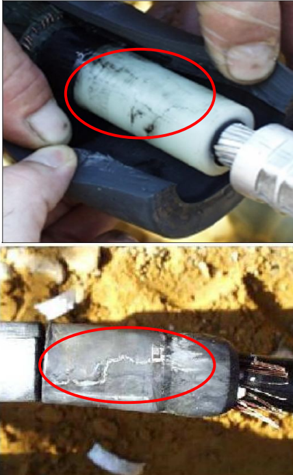
Figure 2.7: A tree like erosion on the surface of polymeric insulation material in a cable joint [5], [13].
