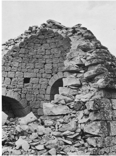
Figure 2.2 Example of partial collapse of Trullo Vault [16]
