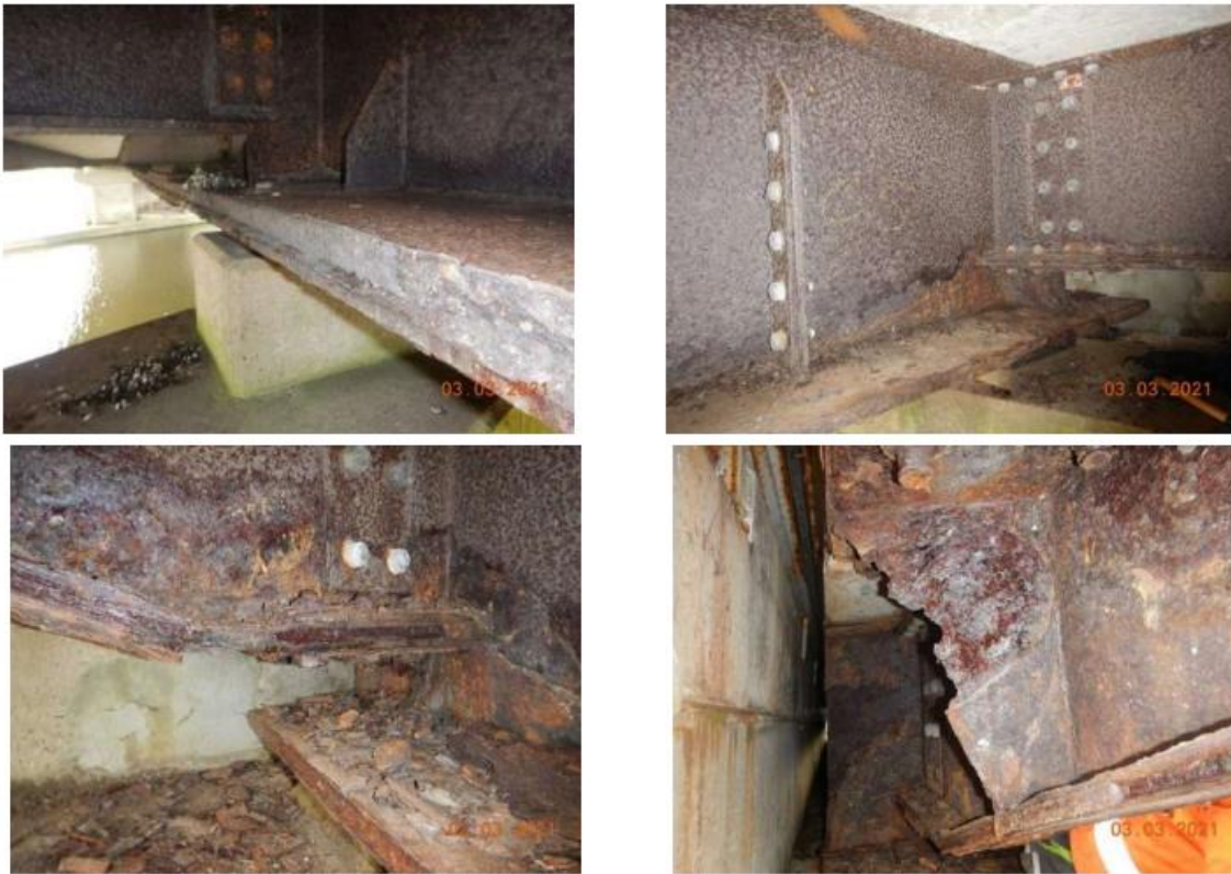
Figure 18 Local significant thickness losses
