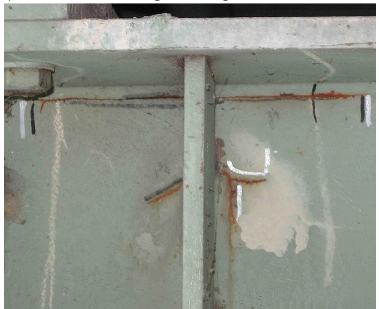
Figure 23 Fatigue cracks on conventional painted steel bridge (Center of advanced infrastructure and transportation, sd)
