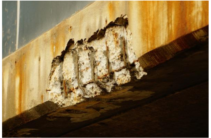
Figure 20 Extreme example of rust stains (shutterstock, 2021)
