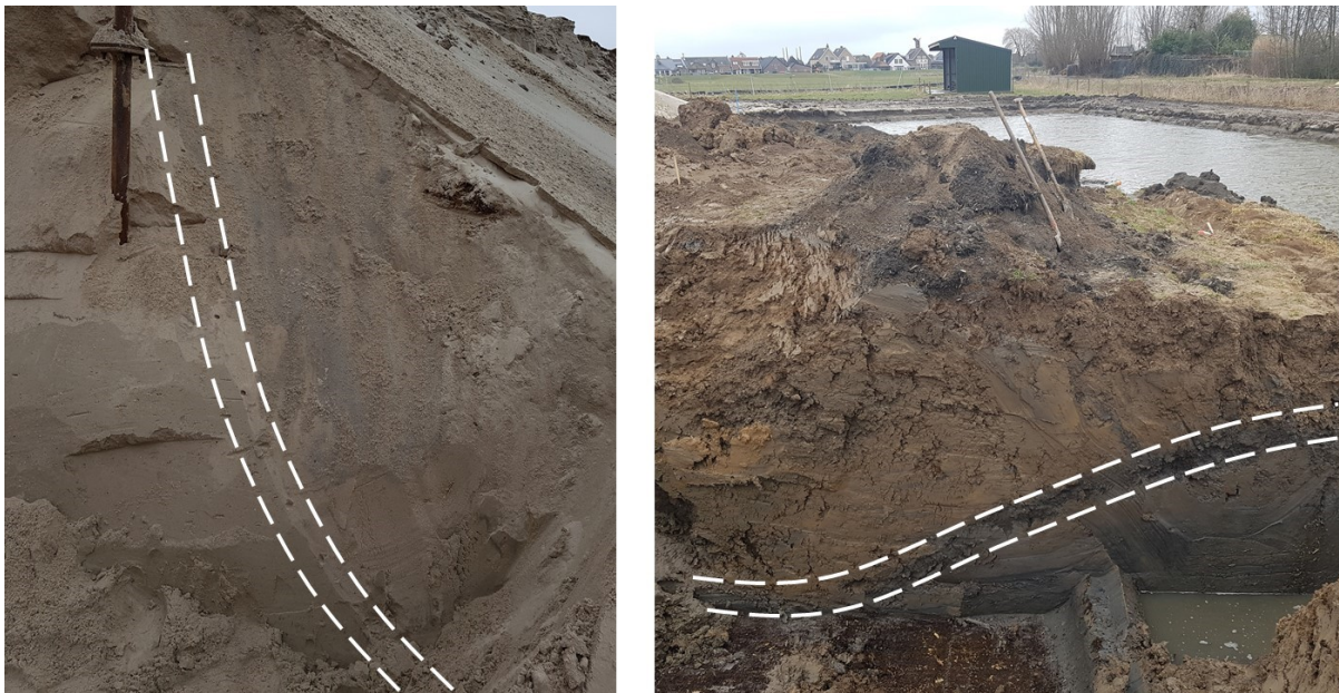
Figure 4.33 Left: Failure surface at the embankment in the sand layer 1a indicated by the dashed lines. Right: failure surface at the toe in soft clay layer 3a just above peat layer 4.
