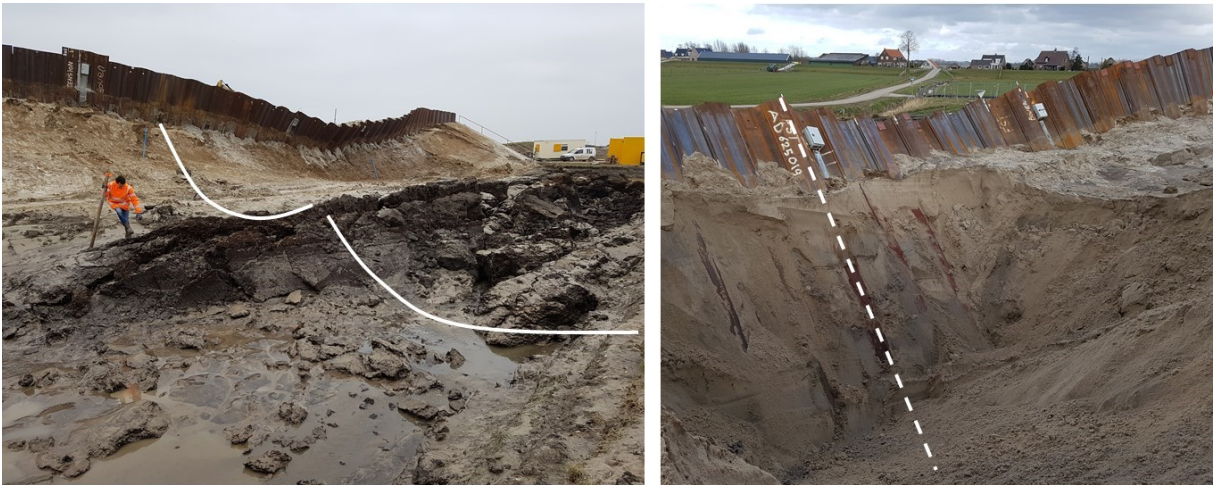
Figure 4.37 Left Side view of the SPD failure mode after draining the ditch, with clear indication of the exit point of the slip circle. Right Top/back view of the sheet piles after failure and local excavation, the dashed line indicates the inclination of the sheet pile. All interlocks of sheet piles are still intact.
