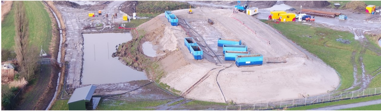
Figure 4.32 Areal view of the Eemdijk test embankment with the failed slope of the GD on the left side (February 2018). The total length of the sliding wedge is about 30 m. The sheet piles and the ditch of the SPD at the right side are not yet present. [Photo courtesy https://www.hwbp.nl/kennisbank/pov-macrostabilititeit ].
