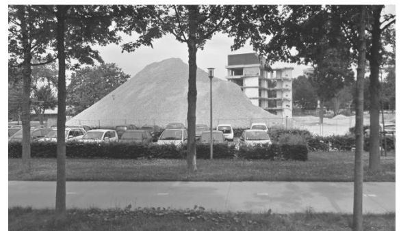
Figure 6: Demolition of Mondrian Care Home in Heerlen generates vast amounts of concrete debris.
