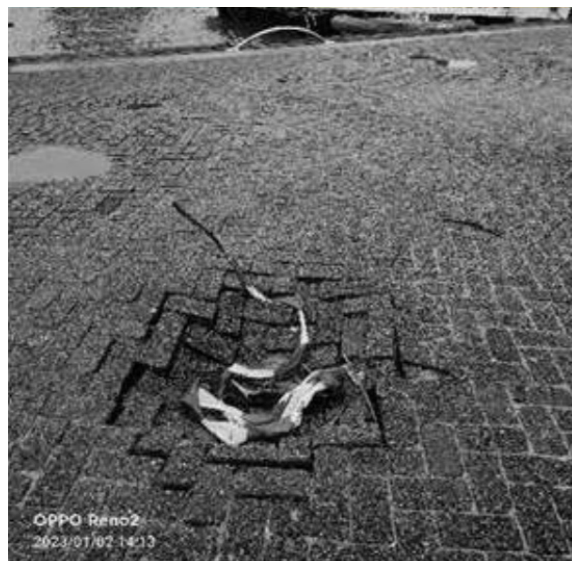
Figure 21 – Sinkhole Caused by Failure (CROW)
