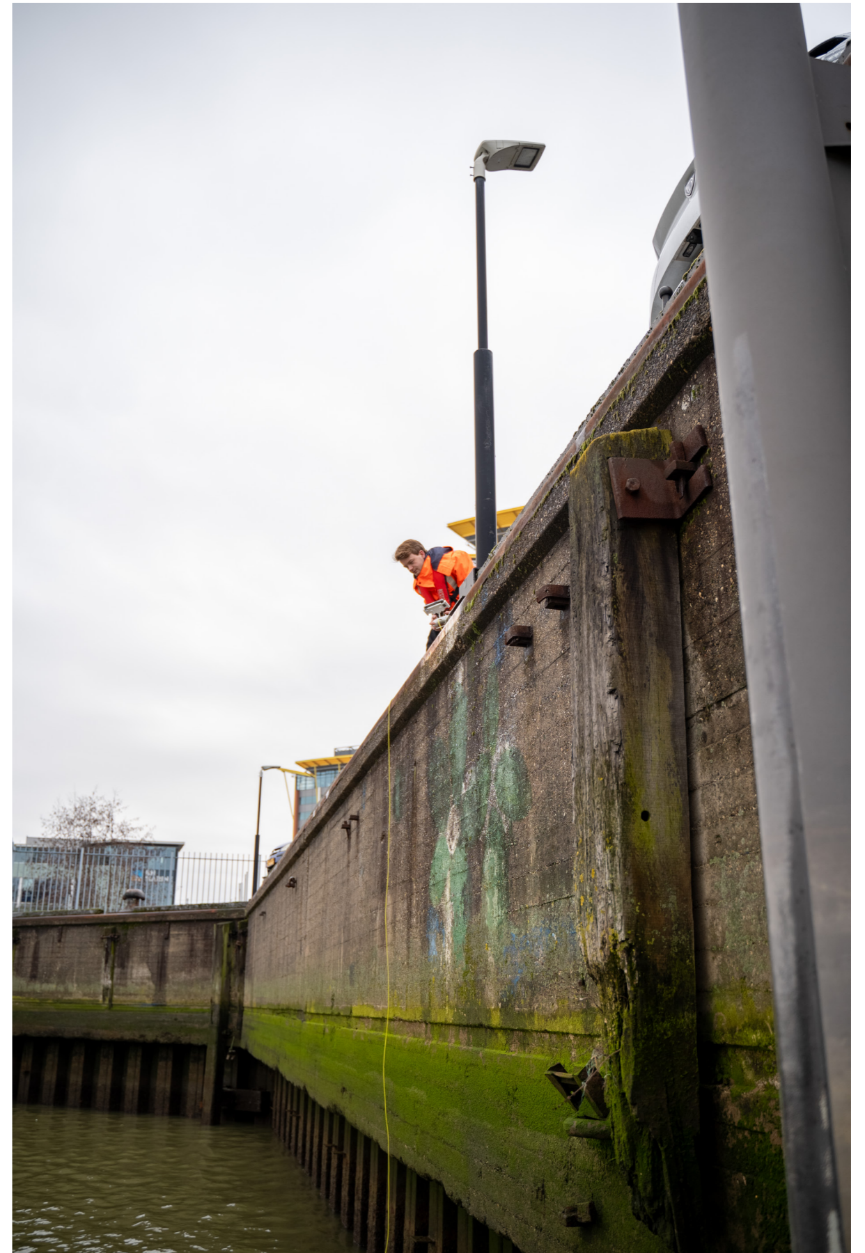
Figure 30 – Dummy inspection illustrating concrete overhanging sheet pile.
