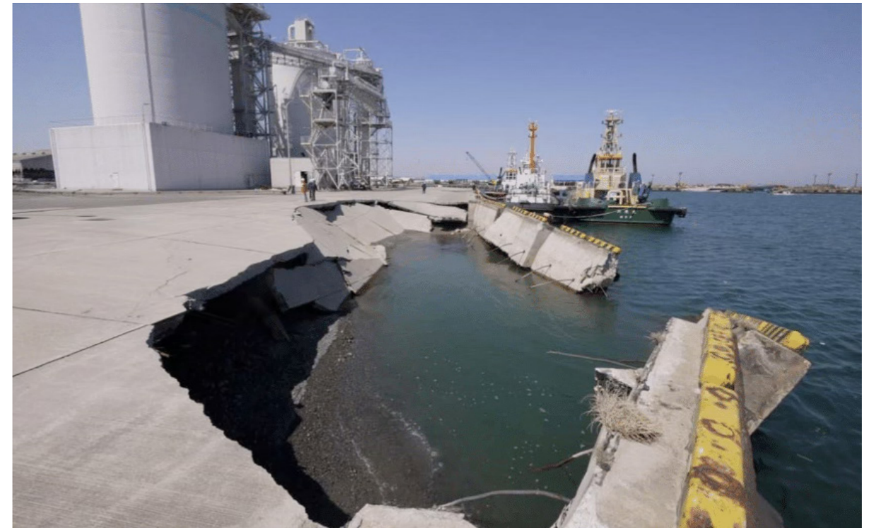
Figure 23 – Quay Collapsed due to Sheet Pile Failure
