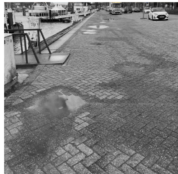
Figure 22 – Sinkhole Caused by Failure (CROW)
