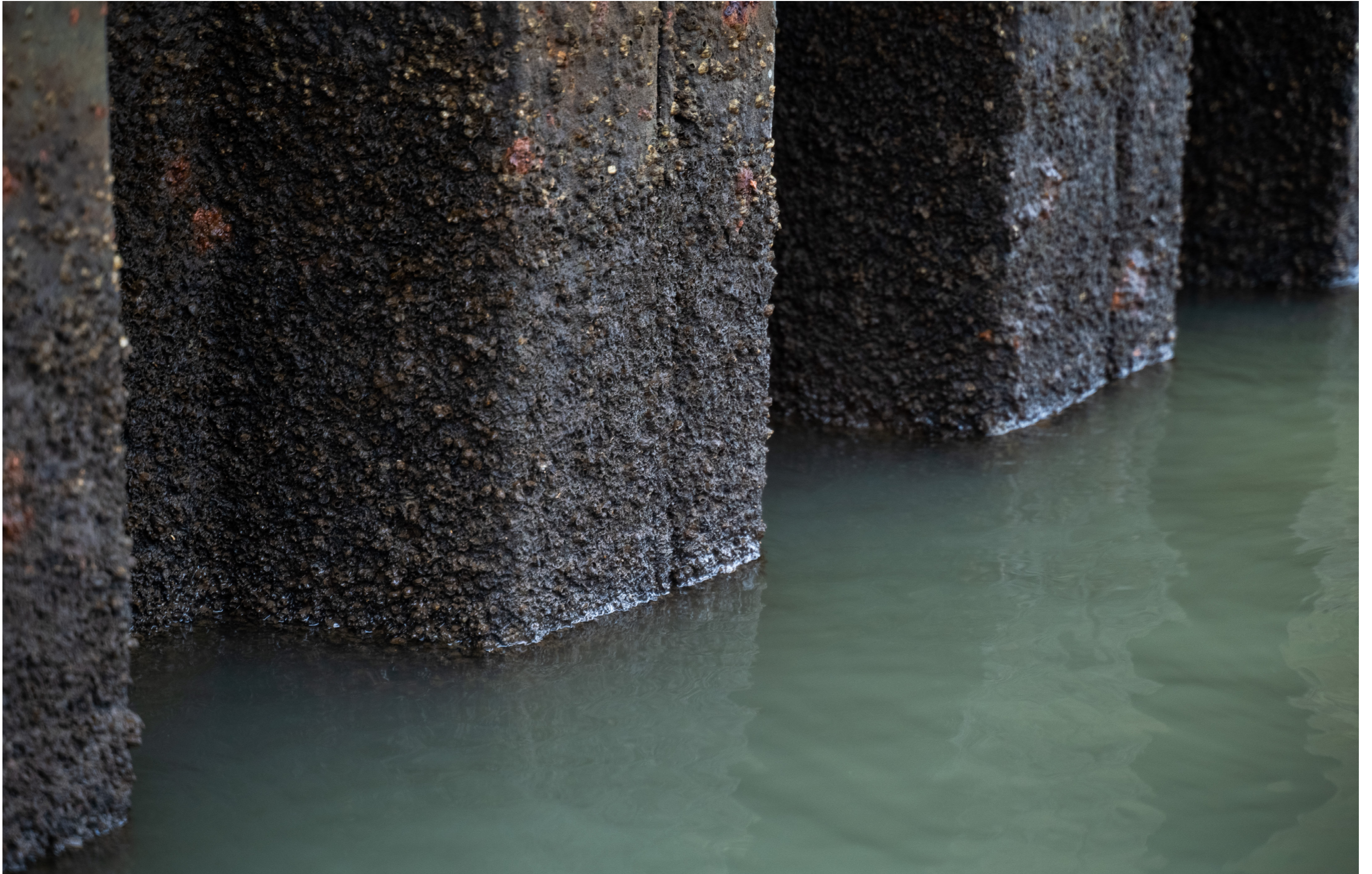
Figure 6 - Sheet Pile with Marine Growth
