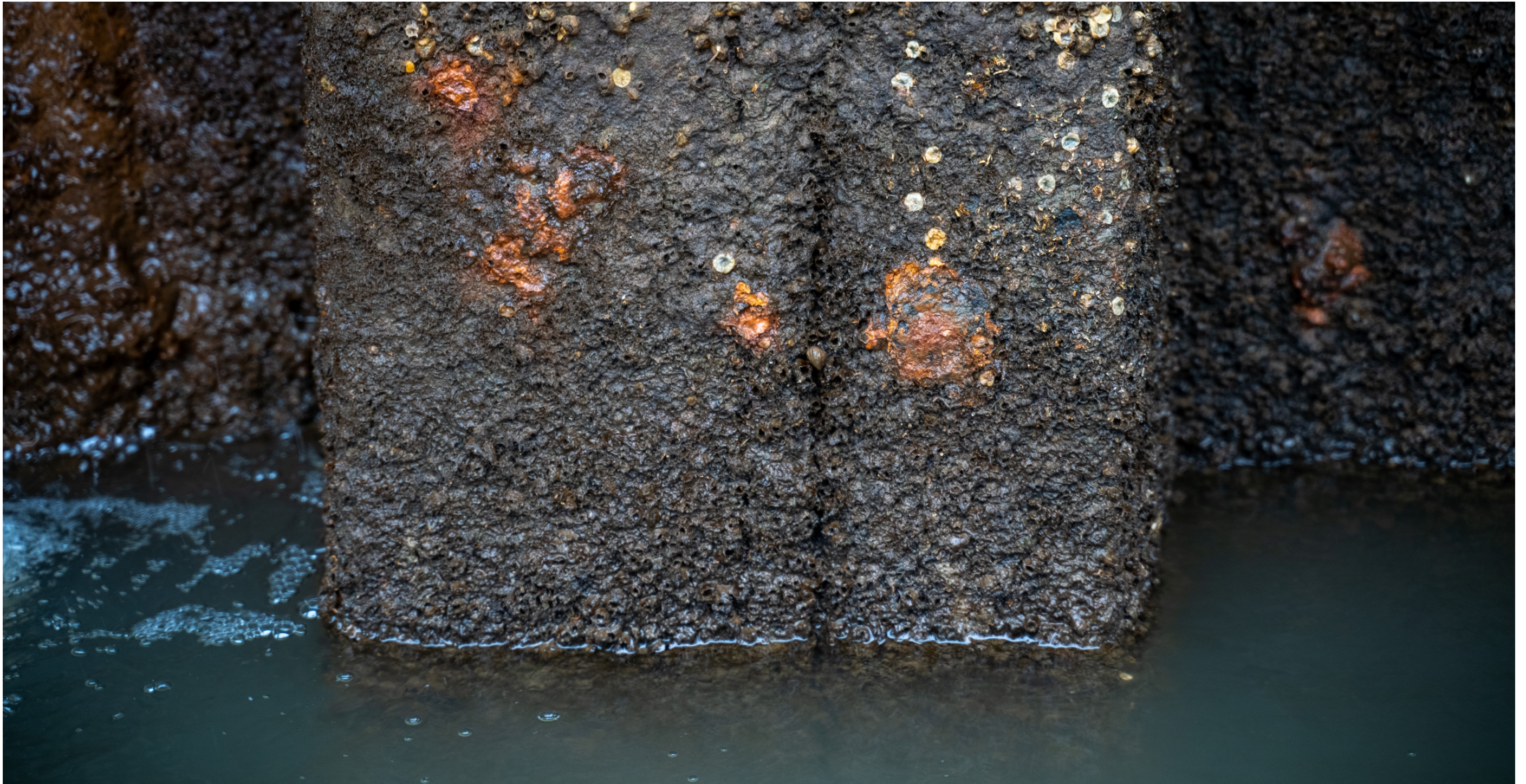
Figure 20 – Corrosion on Sheet Pile
