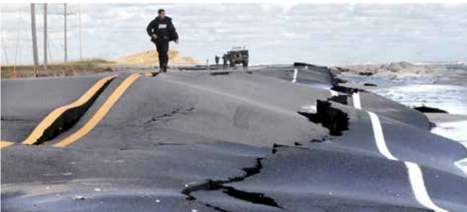
13 Damages in Coney Island © NYT
