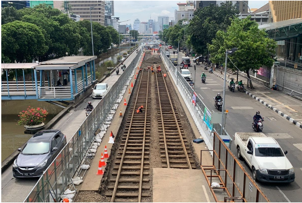
Figure 17. The old tram rails built in Dutch colonization period was covered by post-colonial government of Soekarno and was re-discovered during the construction of Jakarta MRT in 2022. On Kompas.com, 2022.
