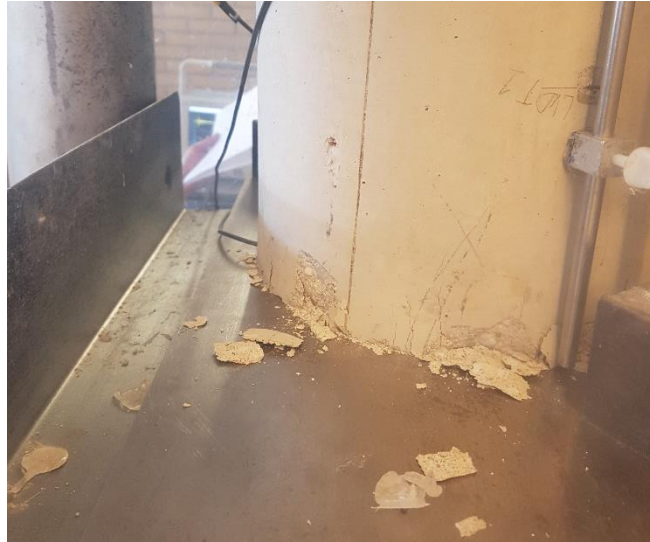
Figure 5.31. Spalling at the base of the specimen, noticed after the third loading part of the first day.
