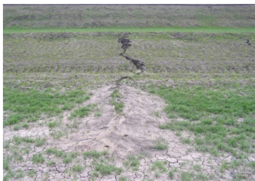
Figure 1. Soil grains washed out from the dike
