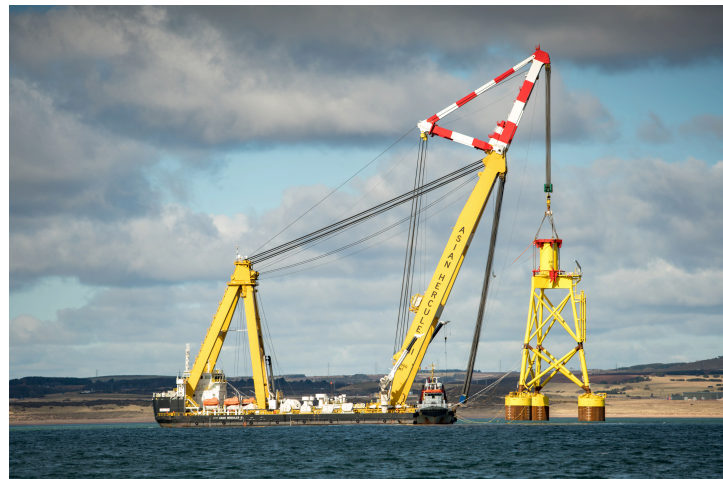
Aberdeen SBJ installation
