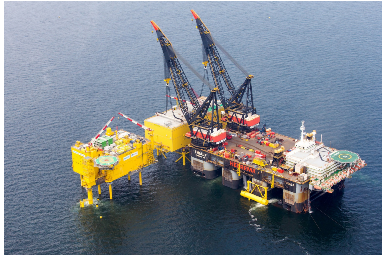
Figure 3.1: Offshore wind power converter station installation on a jacket by the HMC Thialf (HMC, 2015)
