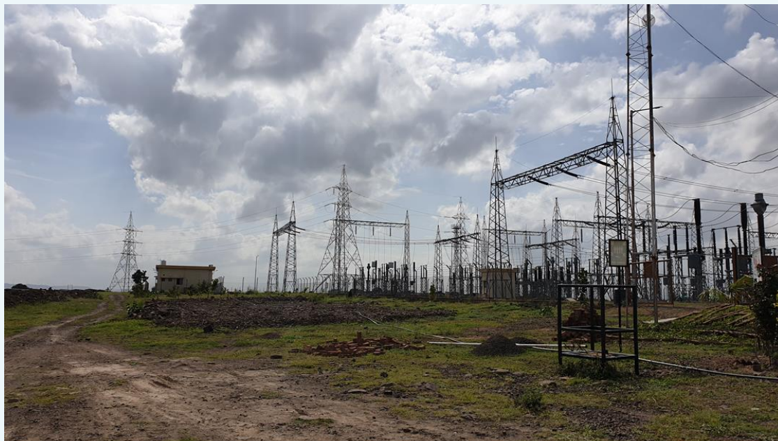
Fig 5.3 : Company substation (Source: author)
