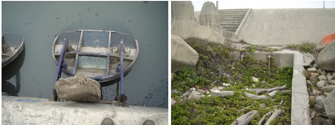
Figure 11.2 An outlet forced open with a stone (left) and completely clogged up with debris (right)
