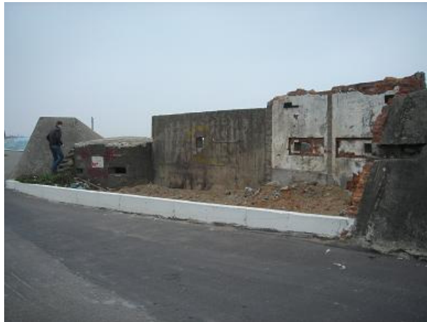
Figure 2.8 Dike interrupted by deteriorated military structure
