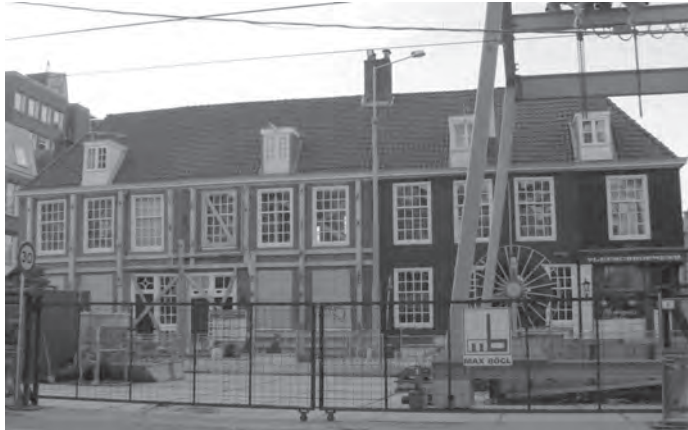
Figure 1.1: Masonry building damaged by differential settlements, Vijzelgracht, Amsterdam. Temporary supporting structures are visible on the left part.
