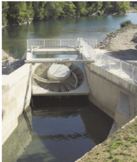
Figure 3-5: Very low head turbine in channel
