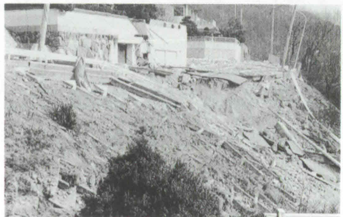
Photo 6 Collapsed embankment at Nishi-okamoto 7-chome
