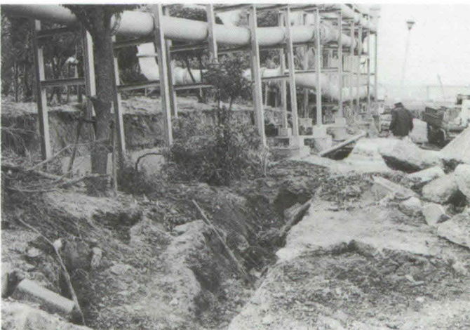
Photo 5 Damaged Higashi-Nada Sewage Treatment Plant
