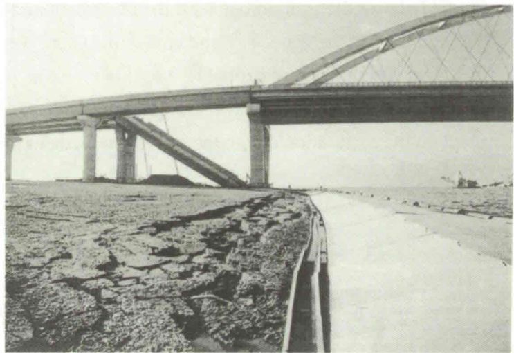
Photo 2 Revetment in front of bridge pier and nearby conditions
