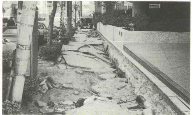
Photo 6 Damage to sidewalk (No. 1)
