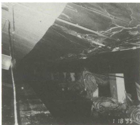
Photo 15 Failure of central subway columns holding up slab of rigid-frame box structure (Taikai Station, Kobe Express Railway)
