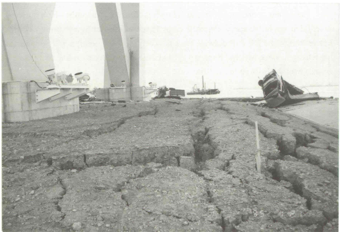
Photo 3 Cracks on the ground around the Nishinomiya Bridge abutment
