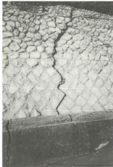
Photo 4 Vertical crack in stone retaining wall
