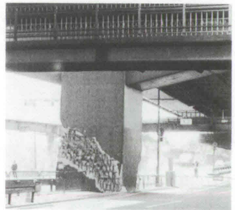
K6: Shear cracking
