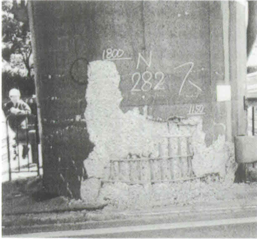
K3: Yielding of reinforcement
