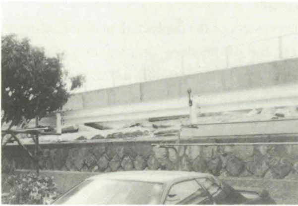
Photo 3 Shorenji River (damage to levee crown)
