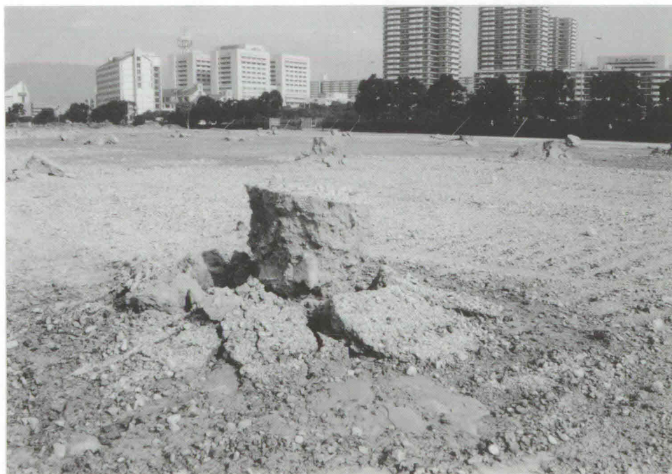
Photo 1 Cast-in-situ concrete pile protruding above ground after settlement of surrounding ground
