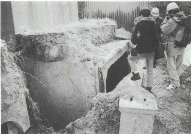
Photo 3 Damaged Higashi-Nada Sewage Treatment Plant
