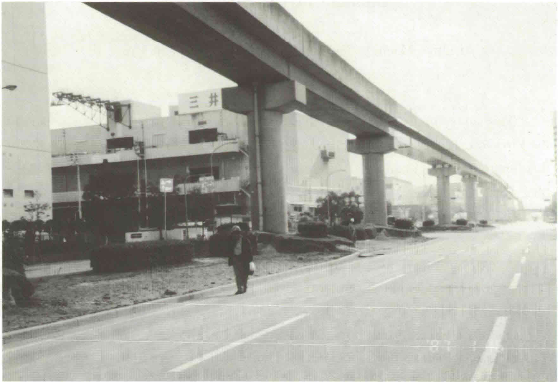
Photo 2 Ground settlement around Shinkansen monorail support column foundations
