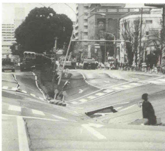
Photo 16 Subsided road surface directly above Taikai Station
