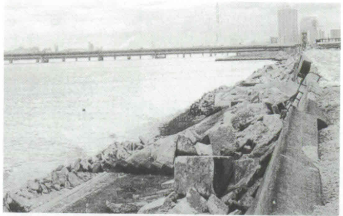
Photo 11 Shinyodogawa river embankment damage
