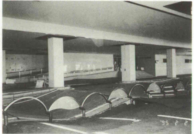
Photo 6 Damage to parking lot above duct route
