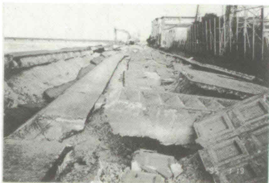
Photo 23 Collapsed levee on the left bank of the Yodogawa river
