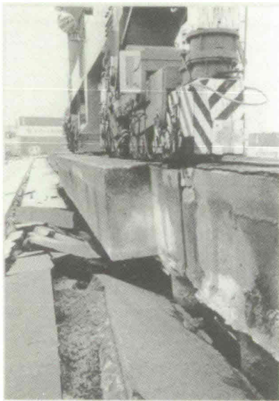
Photo 9 Settled North Wharf
