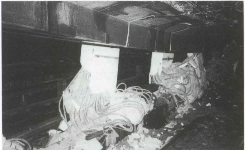
Photograph 5 The columns have collapsed as a result of the progress of the condition shown in Photograph 4
