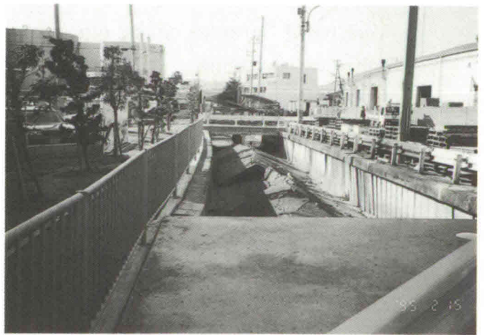
Photo 12 Damage to the concrete riverbed near Nagata Port
