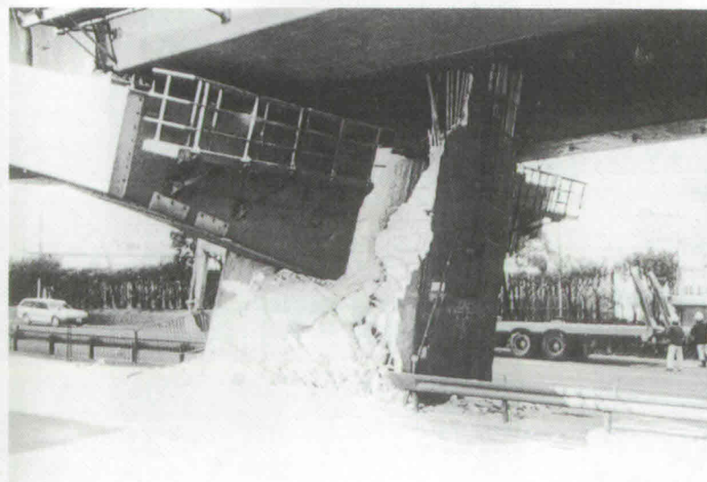
K7: Collapse of single-column rectangular bridge pier
