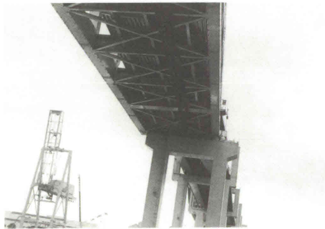
Photograph 15 Transverse movement of girders on Rokko Island Bridge
