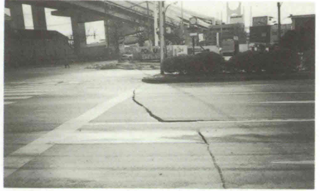
Photo 4 Cracks near intersection (No. 1)
