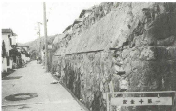
Photo 5 Bulging of two-stage retaining wall
