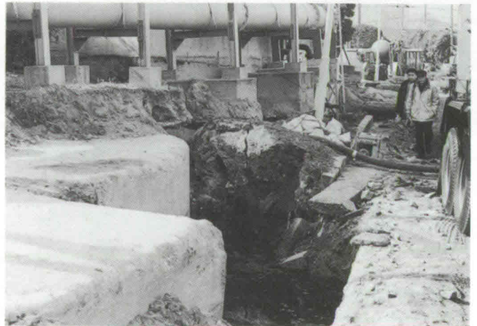
Photo 4 Damaged Higashi-Nada Sewage Treatment Plant
