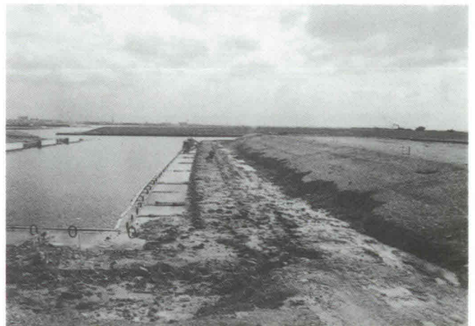
Photo 4 Subsidence of revetments at the site off Minami Ashiya coast
