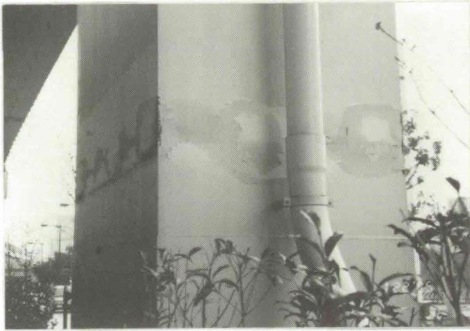
Photo 7 Locally buckled steel pier of rigid-frame elevated expressway (Kobe Route, near Koshien)
