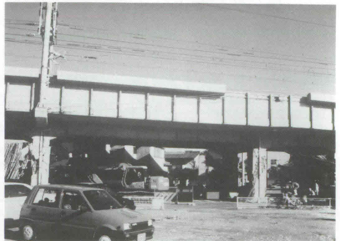
Photo 4 Damage to rigid-frame viaduct with three unequal spans (near Nishi-Akashi Station, Sanyo Bullet Train Line)
