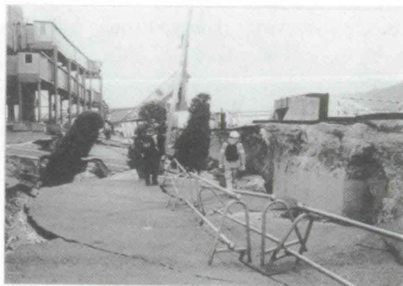
Photo 8 Settled ferry terminal
