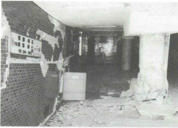
Photo 1 Damage to B1 floor of Daikai station
