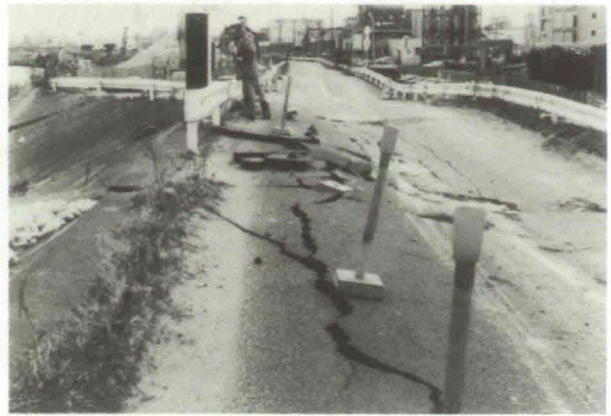
Photo 4 Kanzaki River (cracking and settlement of levee crown)
