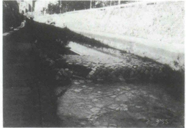
(b) Damaged main channel revetment and consolidation work
