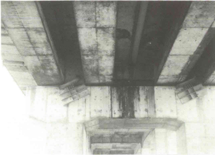
Photo 9 Failure of devices to check the lateral movement of girders (Kaminoro Overbridge, Sanyo Bullet Train Line in Nishinomiya City); failed bolts
