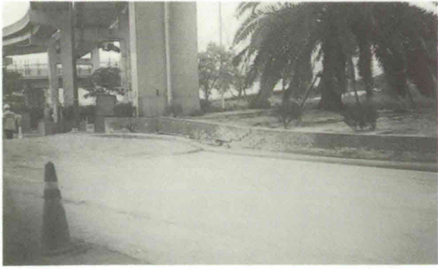
Photo 3 Wavy road surface (No. 2)
