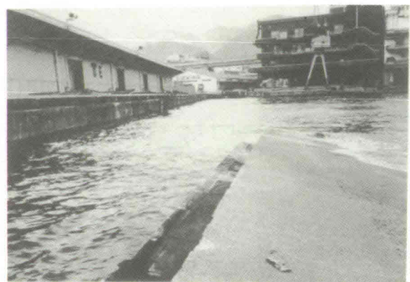
Photo 6 Damaged east quay wall of No. 1 jetty
