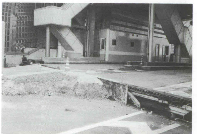
Photograph 10 Drop on the road surface near Minami-Ashiyama Toll Gate
