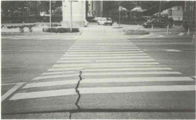
Photo 5 Cracks near intersection (No. 2)
