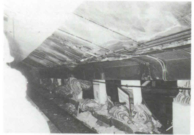
Photo 2 Damage to B2 floor of Daikai station (Nagata-cho side)
