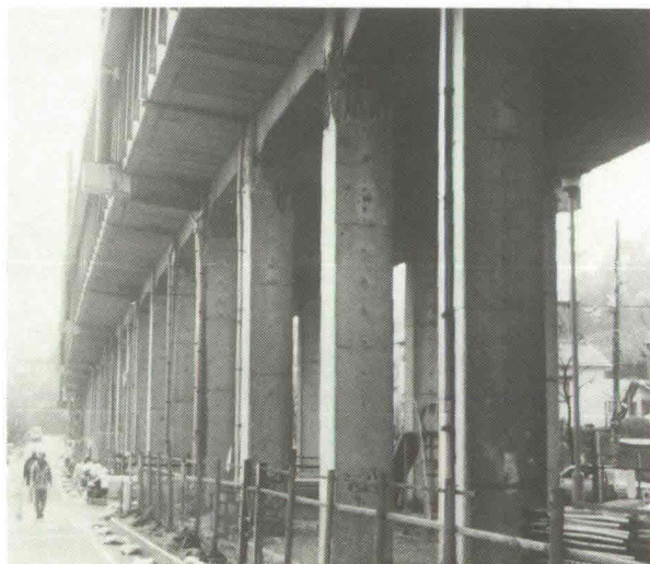
Photo 2 Damage to tops of columns of rigid-frame viaduct, just below haunch
