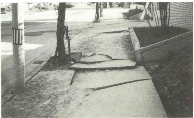
Photo 7 Damage to sidewalk (No. 2)
