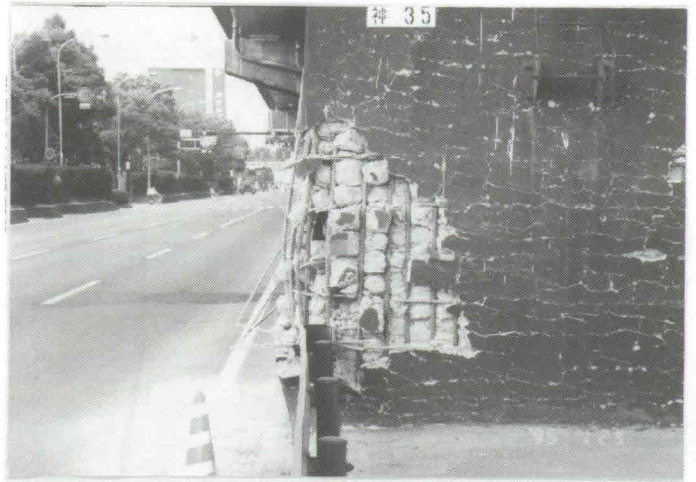
Photo 2 Base fracture in RC pier of elevated expressway (Kobe Route, near Koshien)
