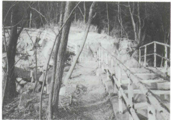
Photo 2 Damaged slope in the Tsuru- kabuto area, Nada Ward
