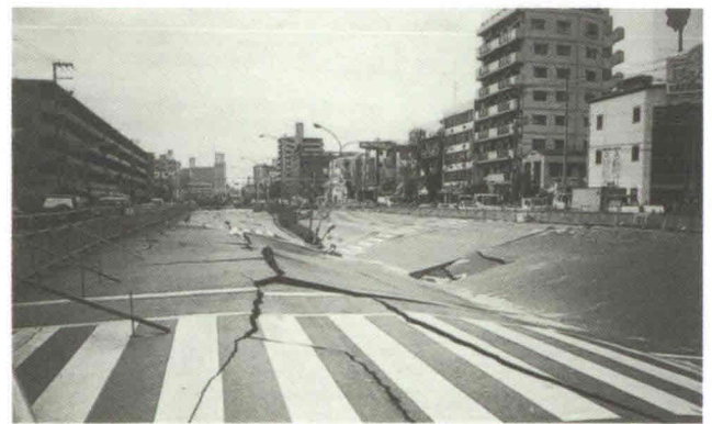
Photo 8 Collapse due to subsidence
