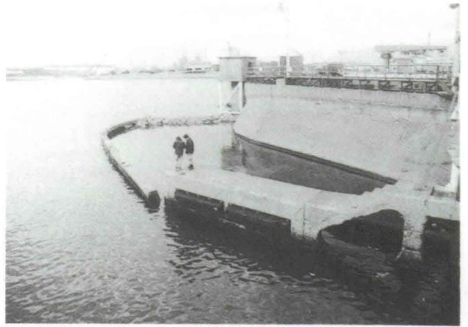
Photo 2 Damage to the Amagasaki Lock
