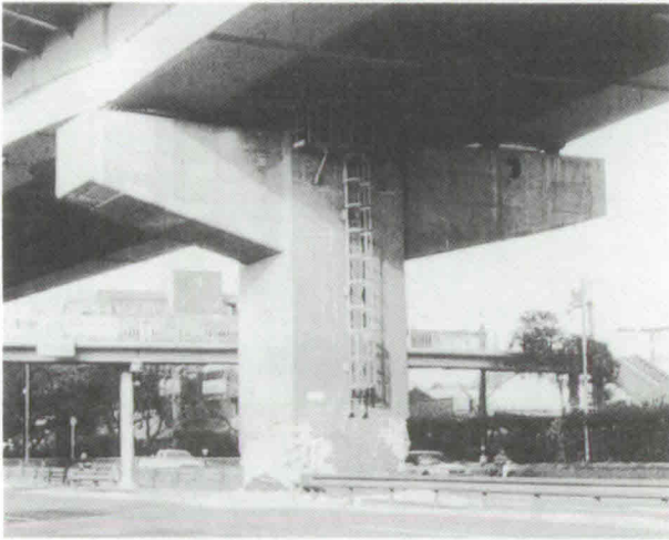
K5: Bridge pier with rectangular section. Flexural yielding.
