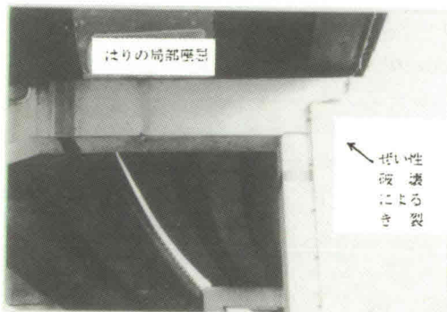
Photo 20 Brittle fracture at a joint between the girder and column on a steel moment frame pier of an elevated road bridge
