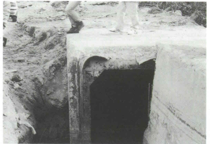
Photo 2 Damaged Higashi-Nada Sewage Treatment Plant
