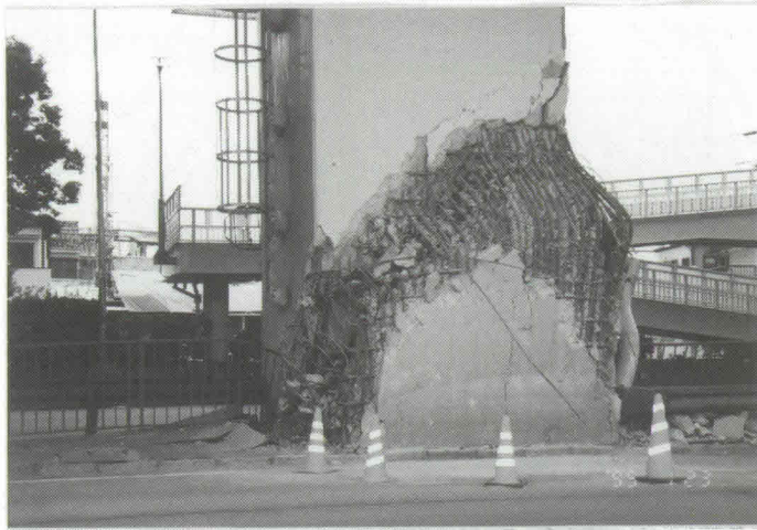
Photo 1 Shear-fractured RC pier on elevated expressway (Kobe Route)
