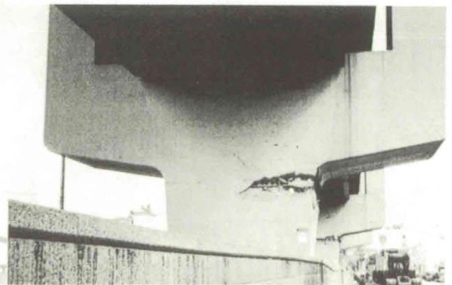
H2: Rebars yielded where reinforcement is reduced
