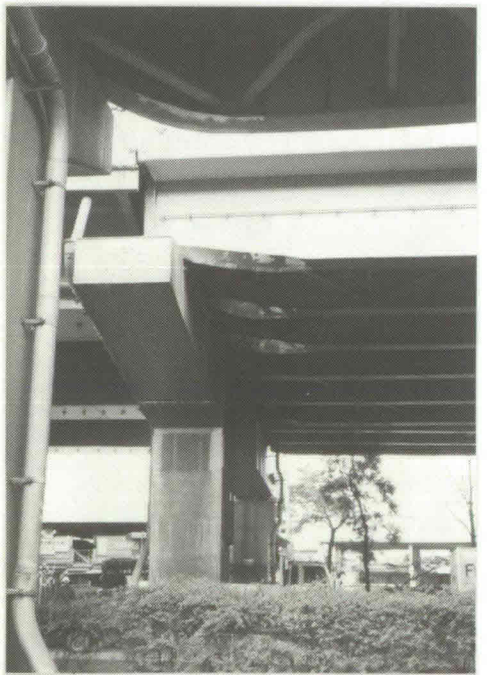
Photo 10 Distorted lower flange due to transverse movement of girder
