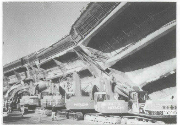
Photo 4 Overturned Pilz-type RC elevated expressway (Kobe Route in Fukae District)
