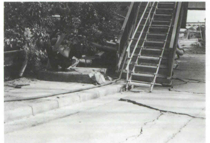
Photo 6 Damaged Higashi-Nada Sewage Treatment Plant
