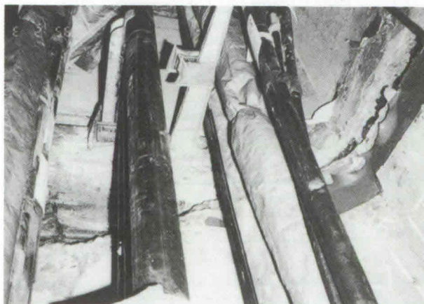
Photo-7 Opening resulting from damage to expansion joint
