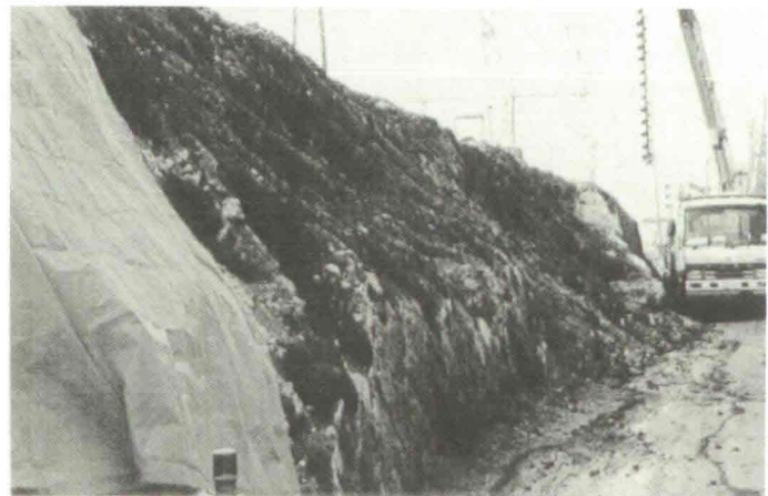
Photo 8 Collapse of fill near Setsumotoyama station
