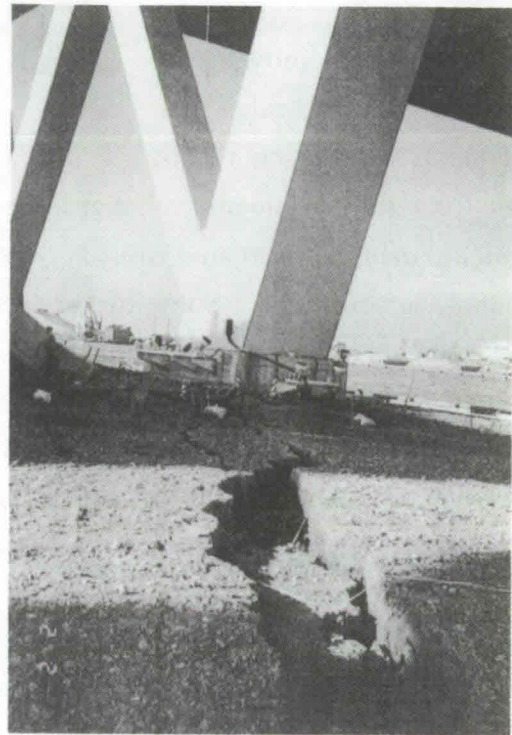
Photo 4 Cracks radiating from bridge pier
