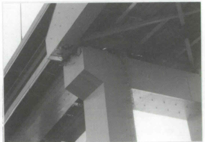
Photo 17 Bridge girder near collapse (Bayshore Route, Rokko Island Bridge)
