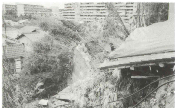
Photo 6 Overturned concrete retaining wall
