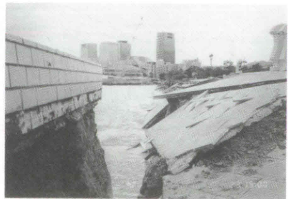
Photo 2 Destroyed south revetment of International Waterfront Park
