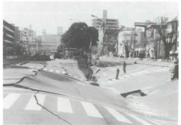
Photo 4 Road subsidence on surface above Daikai station
