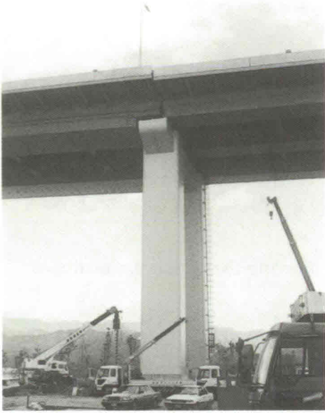
Photo 7 Lateral movement of the foundation of the Hanshin Expressway Wangan Route
