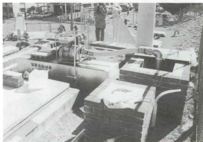
Photo 28 Water supply at distribution yard
