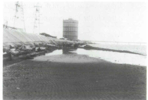
(d) Soil flowing out from embankment structure
