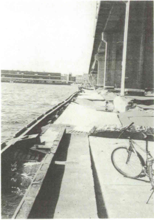
Photo 12 Collapse of southern revetment of the jetty
