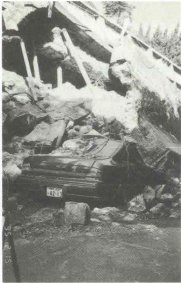
Photo 3 Collapse of stone retaining wall
