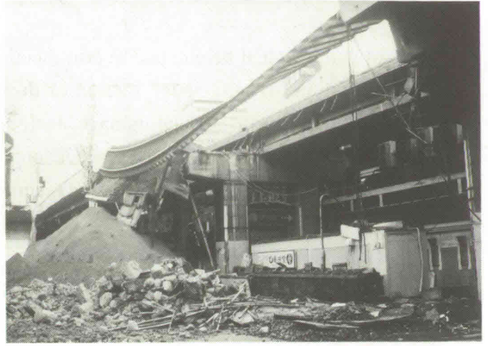
Photo 10 Girders moved laterally and collapsed (near Sannomiya Station, Kobe Express Railway)
