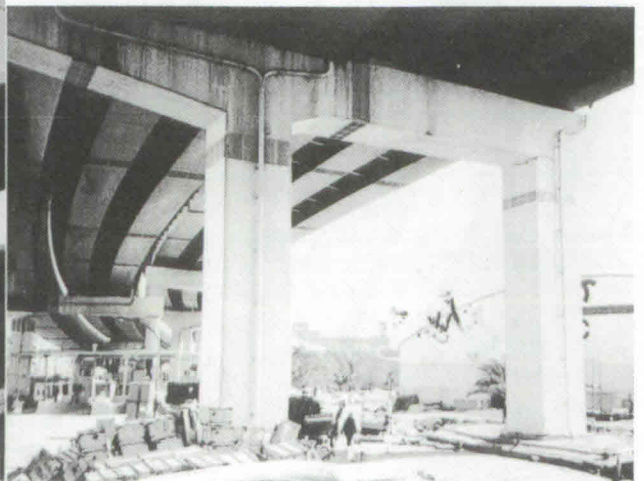
H17: Cracking of steel bridge piers
