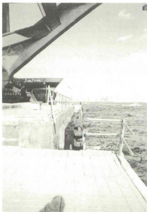
Photo 9 Damage to revetment at foot of the jetty
