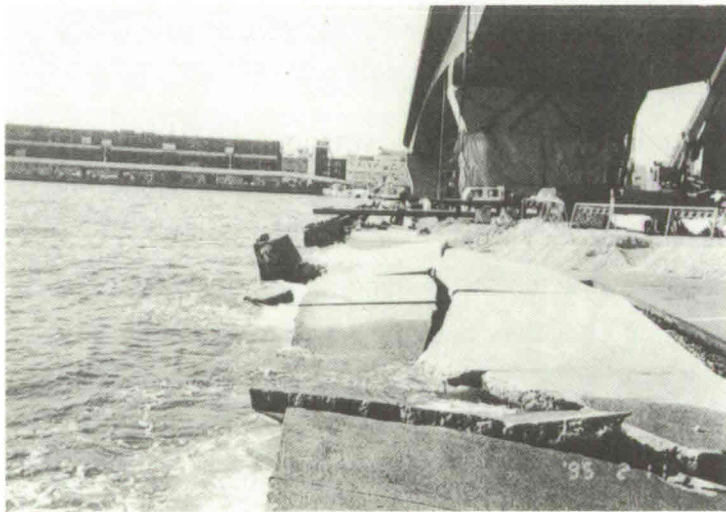
Photo 13 Collapse of revetment of the jetty
