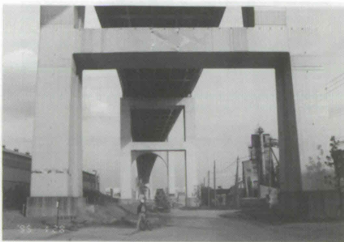
Photo 16 Buckled transverse girder at mid and end piers below fractured Pendel bearing (Bayshore Route, Higashi Kobe Bridge)
