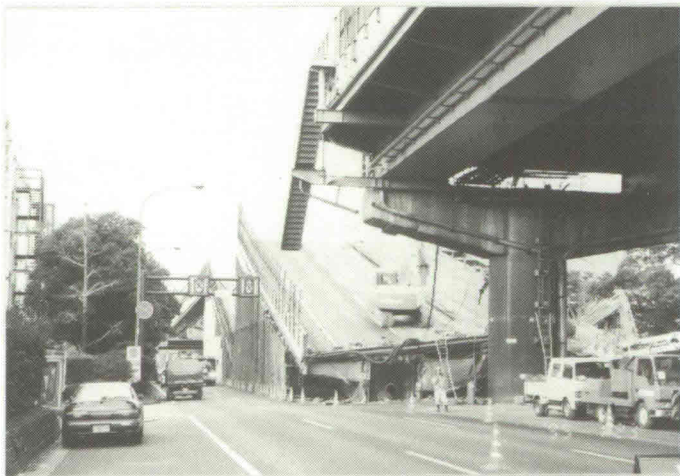
Photo 11 Collapsed expressway girder due to longitudinal movement of girders; device to prevent girder from falling destroyed along with bearings (Kobe Route, at Honcho intersection in Nishinomiya)
