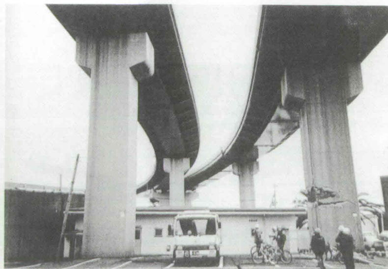
H7: Damage to tall single-column bridge piers. Rebar yielded at point of reinforcement reduction
