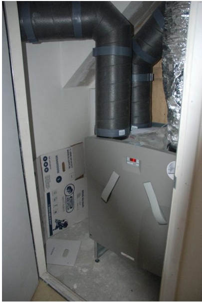
Figure 91. Private home Den Bosch NOM balanced ventilation system
