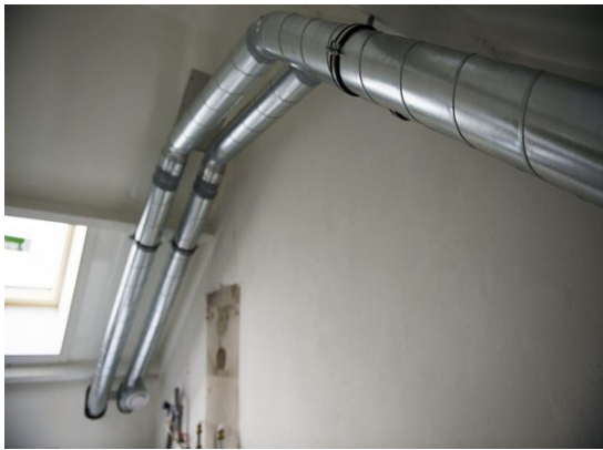
Figure 81. Woonwaard NOM renovation, new ventilation piping + old connections natural gas boiler still visible
