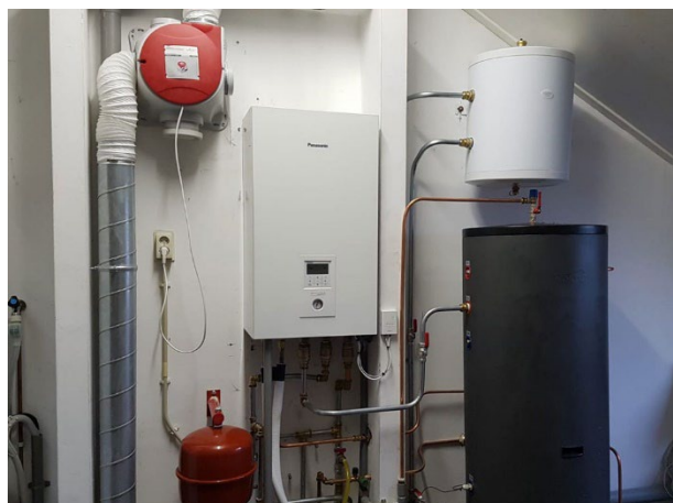
Figure 18. All-electric air source heat pump + DHW boiler + Central heating buffer (panasonicwarmtepompen, 2019)
