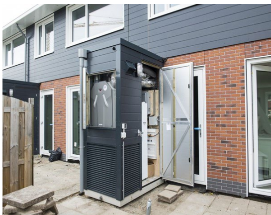
Figure 79. Woonwaard NOM renovation, Building services in extension
