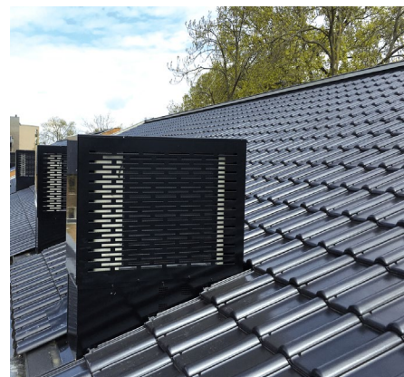
Figure 63. sound-absorbing heat pump housing (HydroCap, 2022)
