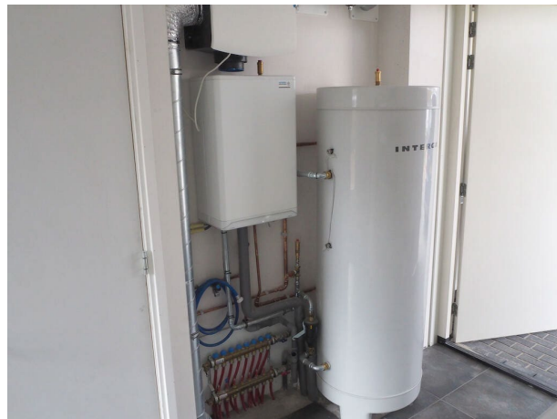
Figure 17. All-electric air source heat pump + DHW boiler (installatiebouw, 2022)
