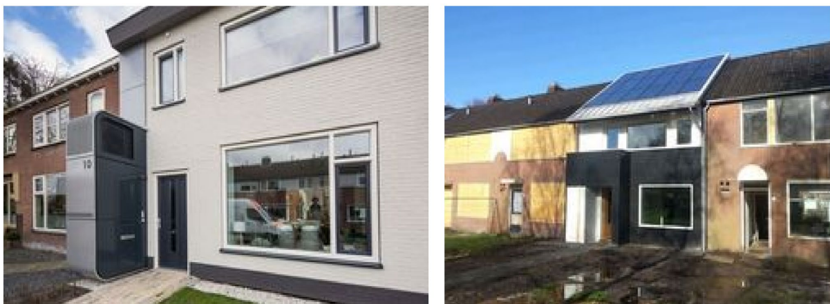
Figure 77. Heating and ventilation installations brought together in a building extension placed outside the dwelling.
