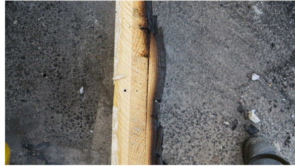
Figure 6.82 Along this edge, up to 3 layers of CLT remain. The inner most layer is almost completely charred.
