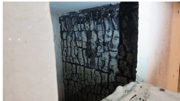
Figure 6.110 The smouldering of the CLT quickly decreased in intensity until no glowing was observed.
