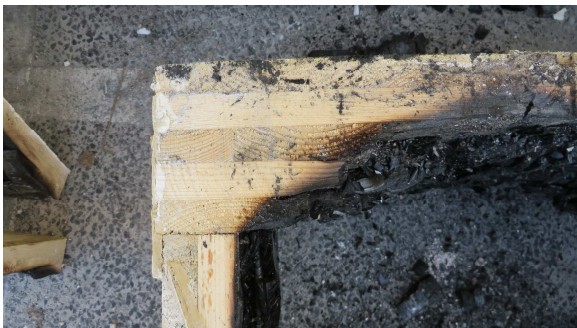
Figure 6.63 In the corners up to 4 layers of CLT were still in place. Beneath the charred out layer, unaffected wood was still present.
