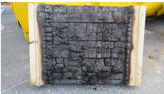
Figure 6.49 Some charred pieces of the first layer are visible, as the charred boards of the second layer.
