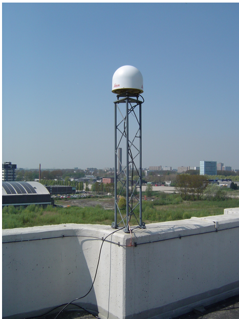
Figure 2. DLF1 high-end Leica LEIAR25.R3 geodetic antenna installed on top of NMI building. Picture is pointing in West direction
