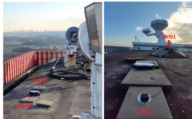
Figure 5. GNSS modules placement on top of EWI building. Left side - installation on the South side of the roof top. Right side - installation on the middle part of the roof top. Both pictures are pointing to the South.
