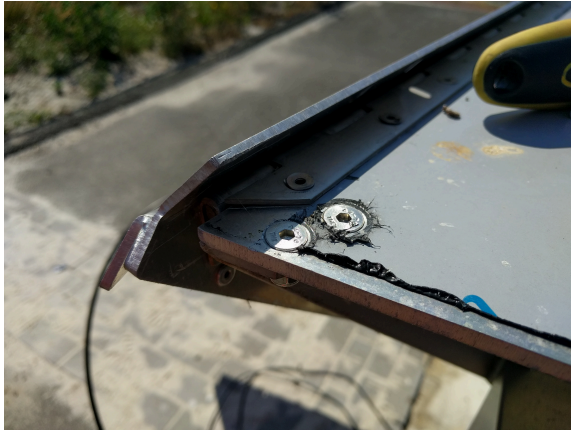
Figure 6.20: Bolts not suitable for levelling.
