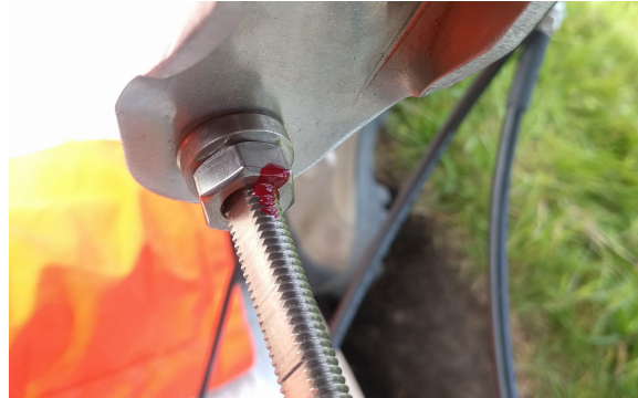
Figure 6.23: Bolts are sealed with a red seal to indicate change.
