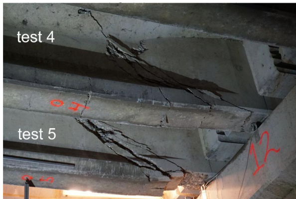
Figure 16. Flexural shear failures in test 4 and 5 (Ensink et al., 2024).
