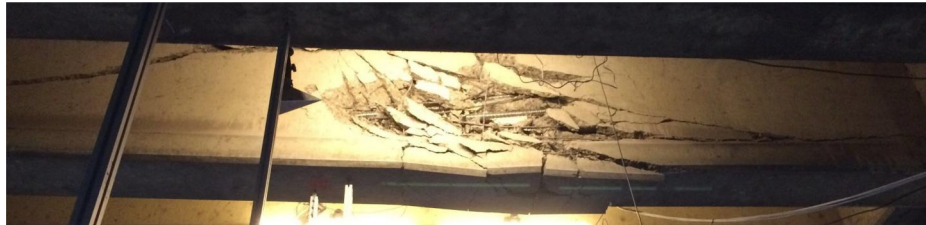
Figure 14. Shear failure of T-girder in test 1. The crossbeam is located on the left side and the end support on the right side (Ensink et al., 2024).
