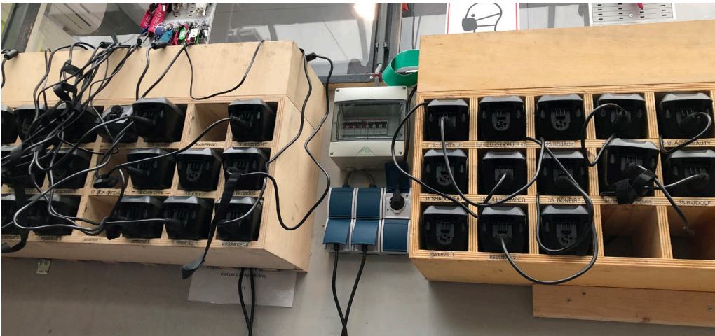
> Figure 26: Custom made charging cabinet at Marleenkookt, built by a local carpenter.
