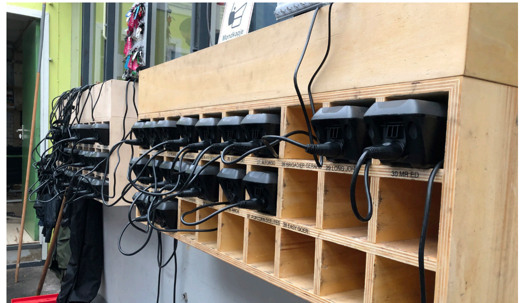
Figure 40: Custom made charging cabinet for around 40 cargobikes at Marleenkookt's main location in Amsterdam. Each battery has a dedicated bike it belongs to, hence the names and
