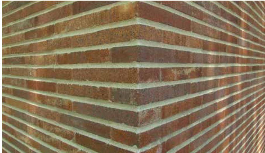
FIG. 2.21 Robie House. Masonry of 'Roman bricks'; deepened horizontal joints, vertical header joints set flush with the face of the bricks and coloured red. [Photo: Mike Sirotnin]
