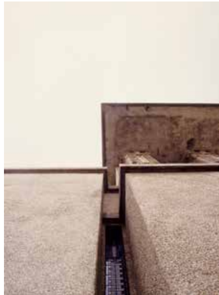
FIG. 1.6 Unity Temple. Slot and 'ladder window' cutting open the shield of the wall. [Photo: Frans Sturkenboom]
