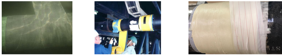
(a) Repair by wrapping of flexible FRP composite [Green, 2010]. (b) Repair by ClockSpring sleeve mechanism [ClockSpring, 2019]. (c) Repair by water activated FRP wrapping [ClockSpring, 2019].
