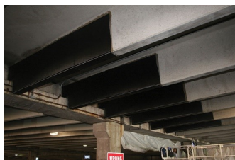
(b) Shear strengthening of parking garage floor [Alkhrdaji, 2018].
