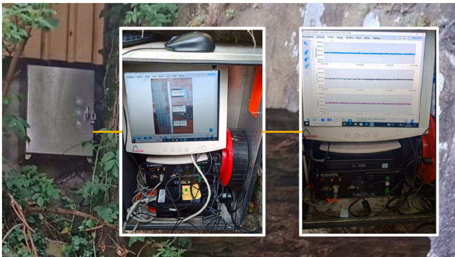
Fig. 5. Steel cabinet showing data acquisition equipment layout.
