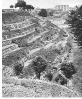
Fig. 2.17 Various progress pictures of the construction of Monte Stella (Archivio Piero Bottoni, 1951-57)
