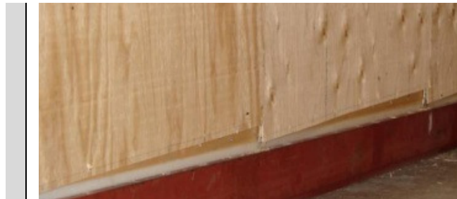
figure 56: Rotation of the sheathing panels can become quite high at ultimate load. (Ni et al., 2010)
