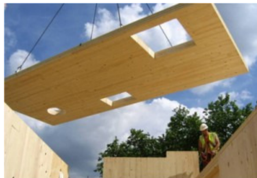
figure 11: Construction using cross-laminated timber: sawn plate elements, structure to be finished at the building site.
