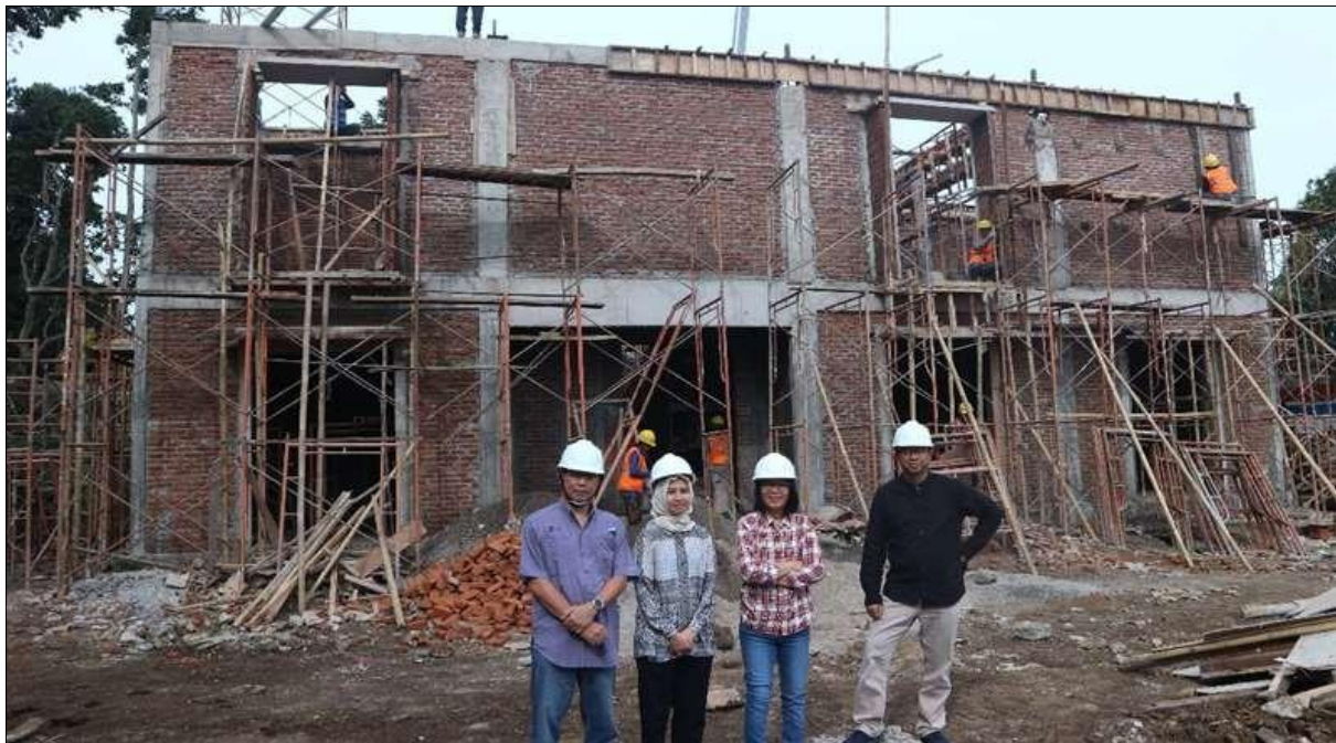
Figure 19: The VGOS telescope tower building (top) and its supporting building (bottom) under construction at Bosscha Observatory in January 2025 (photographs: the authors).
