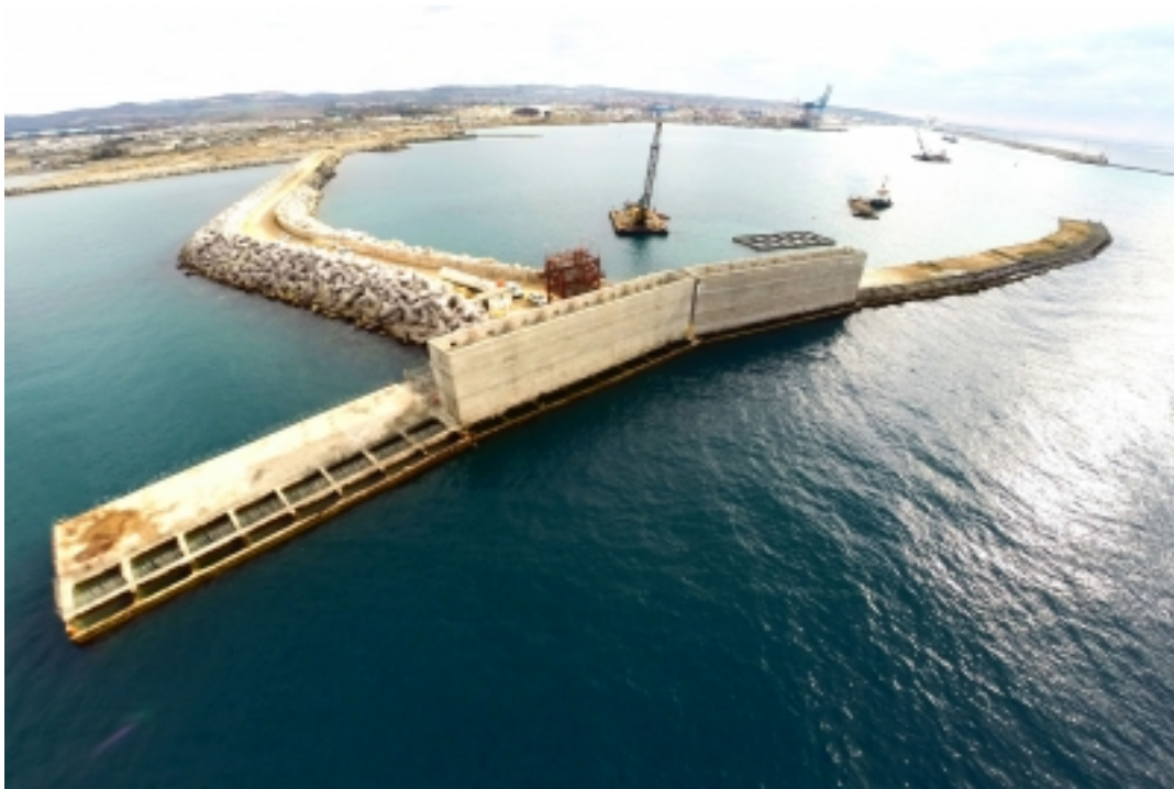
Figure 2.2: The new breakwater of the port of Civitavecchia during construction, showing the individual caissons. [21]
