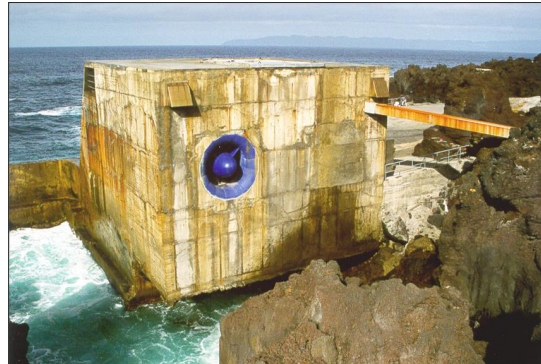
Figure A.4: OWC built on Pico, one of the islands of the Azores, Portugal.
