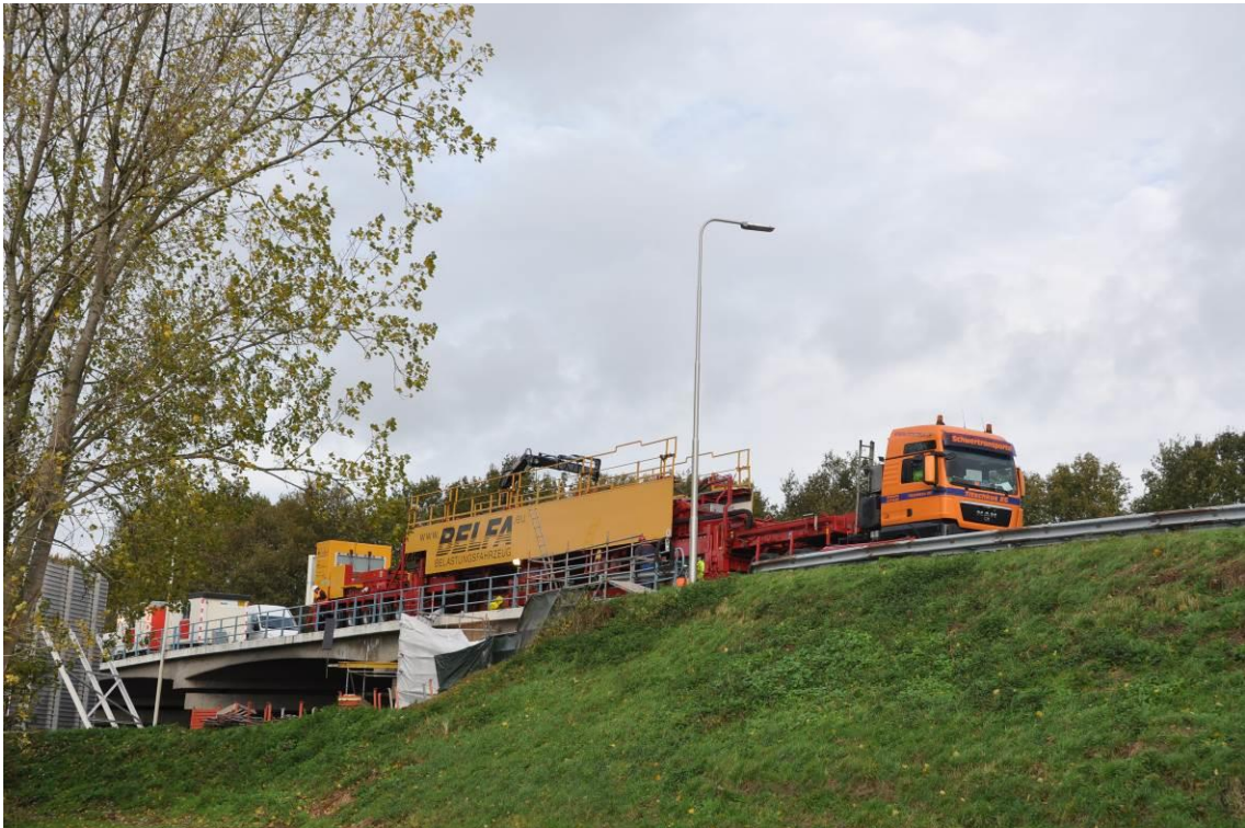
Figure 14. Example of application of load with load testing vehicle. Photograph by D. Hordijk. Printed with permission.
