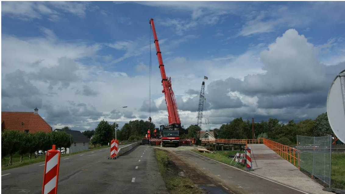
Figure 16. Overview of traffic situation during a load test. From left to right: one lane open for traffic, one lane used for load testing, temporary bike bridge. Photograph by S. Fennis. Printed with permission.
