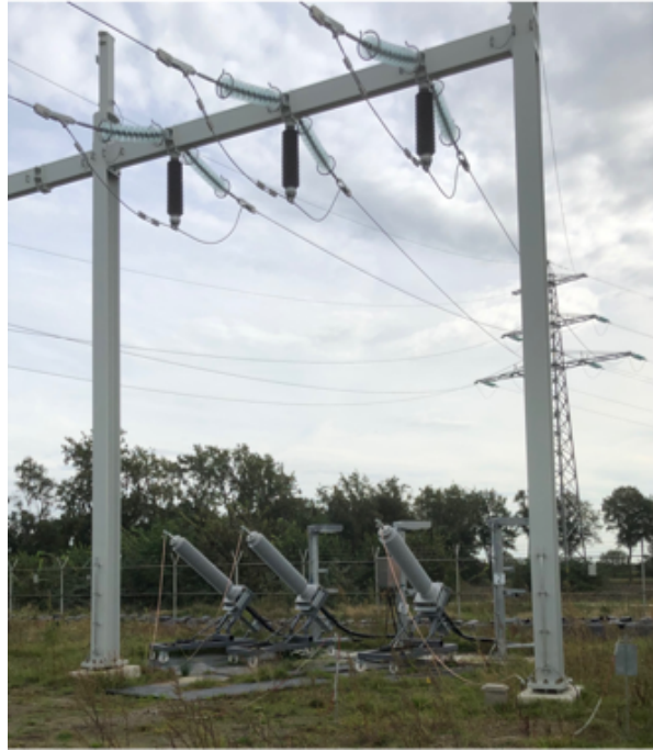
Figure 8.7: Cable end terminals to connect the mobile substation to gantry structure, photo by TenneT.
