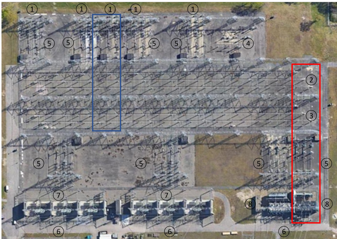
Figure 2.1: Aerial view of the TenneT substation Eindhoven 380.
