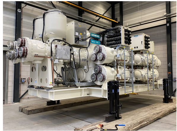
(b) Picture of mobile GIS skid from TenneT (170kV)
