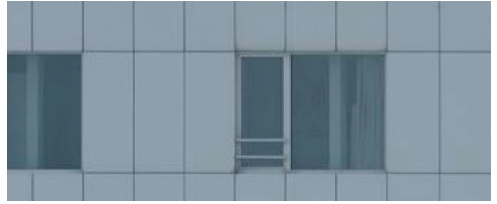
Figure 8.3 | Close-up of the part of the facade of the Montevideo with the light grey cassettes | Source: (Mecanoo 2021)
