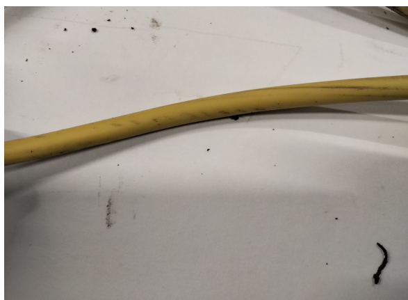
(a) Single conductor from a failed cable on field
