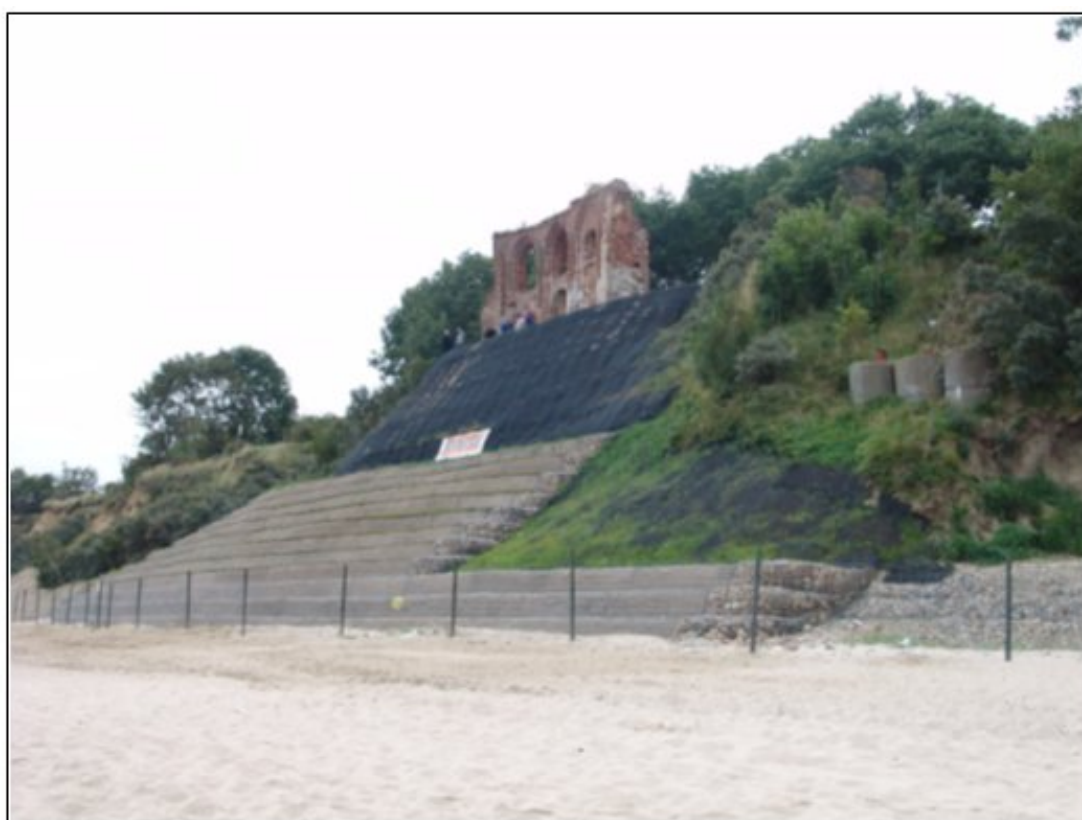
Fig. IV-61. Last combined protection system, achieved in summer 2005.
