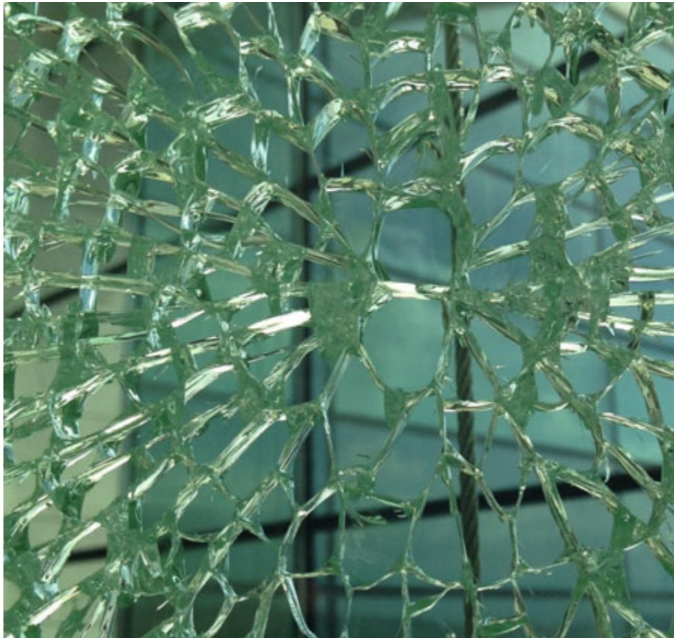
Figure 2.19: Typical fracture pattern in tempered glass due to NiS inclusion (Belis et al., 2019)
