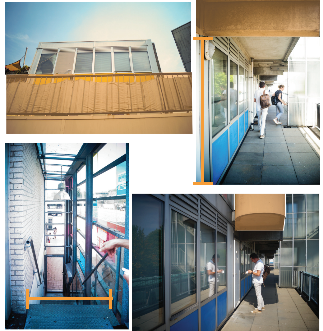
Figure 6.5: Renovation boundary conditions: (Own figure)
